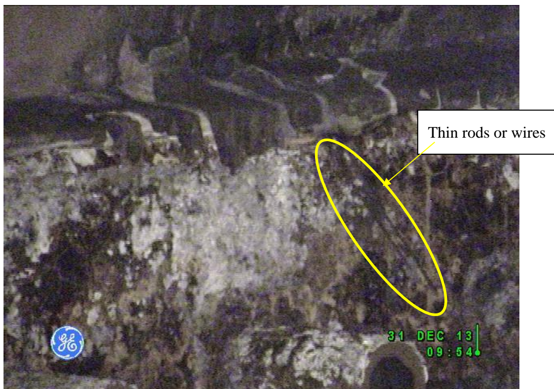
Figure 16 Closeup #3 of Anomaly on Tank T-111 East Wall, December 31, 2013
