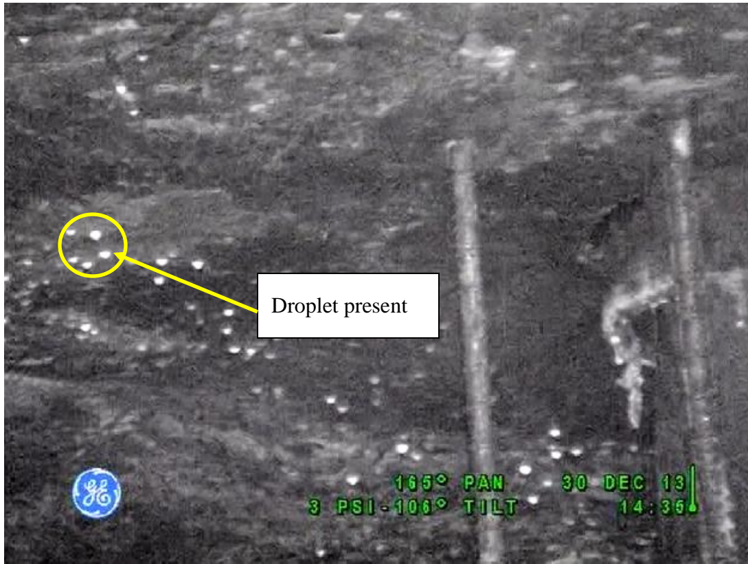
Figure 18 Water Drop from Tank T-111 Dome
