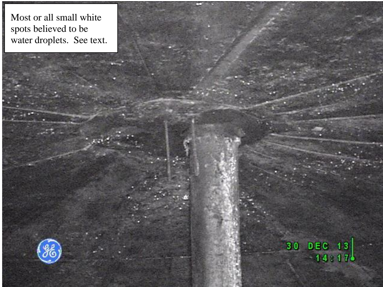
Figure 17 Tank T-111 Showing Water Droplets on Central Dome Area, December 30, 2013
