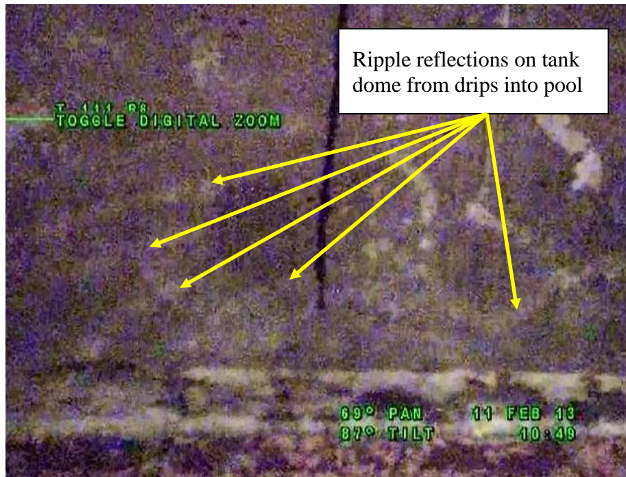
Figure 10 Reflections of Drip Ripples from Pool onto Tank T-111 Dome
