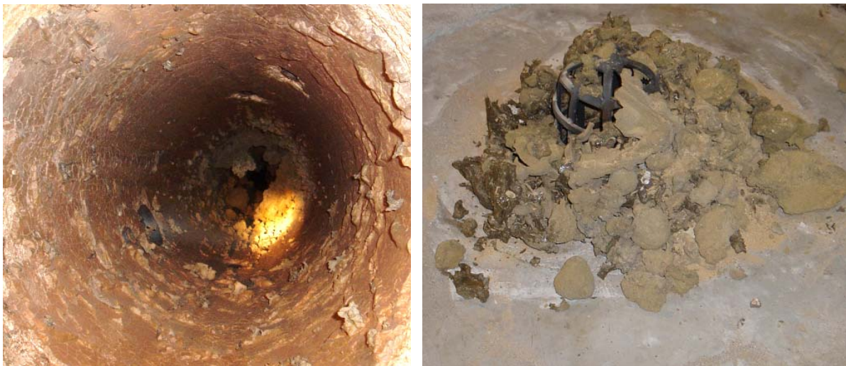
Figure B-9 – Slag Build-up in the Oxidizer
