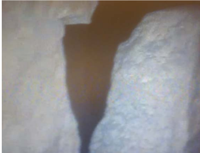
Figure B-12 – Cracks in the Refractory Tiles in the Oxidizer
