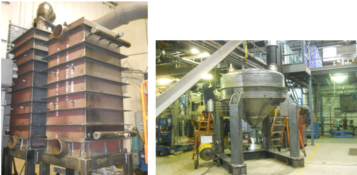
Figure 5-16 – Product Gas Condenser (left) and Reducer Chamber Pot (right)
