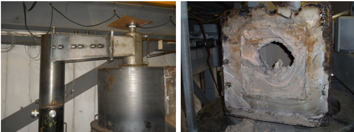
Figure B-7 - Location of Water Leak in Reducer Secondary Cyclone Outlet duct
