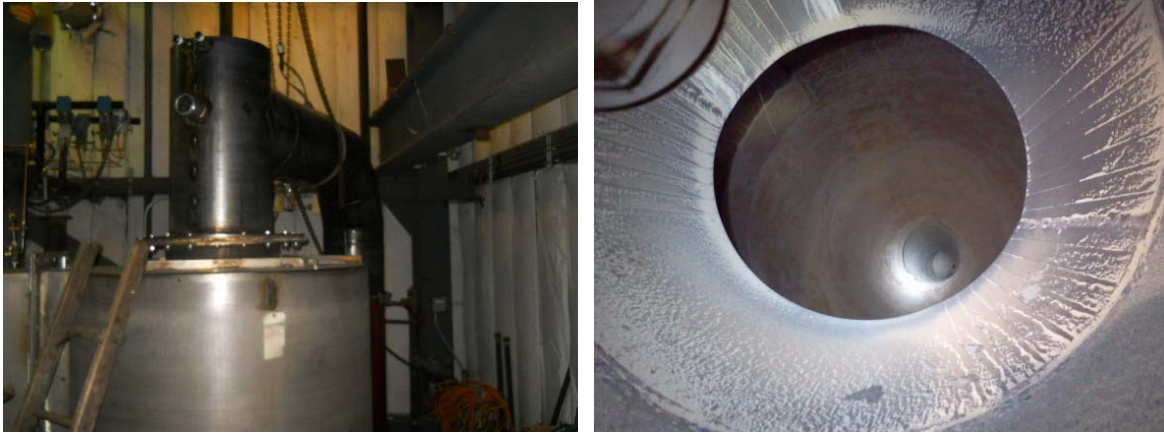
Figure B-6 - Location of Water leak in Oxidizer Cyclone Outlet Duct
