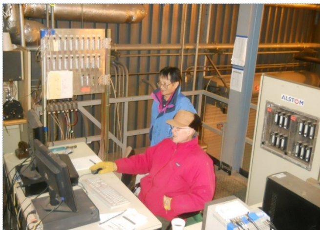
Figure 6-5 - Control Console for the CFM
