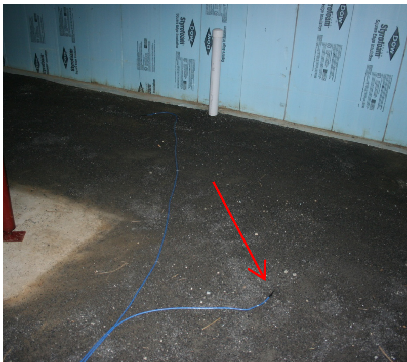
Figure 8. Typical TC installation for measuring soil temperature directly below the slab insulation
