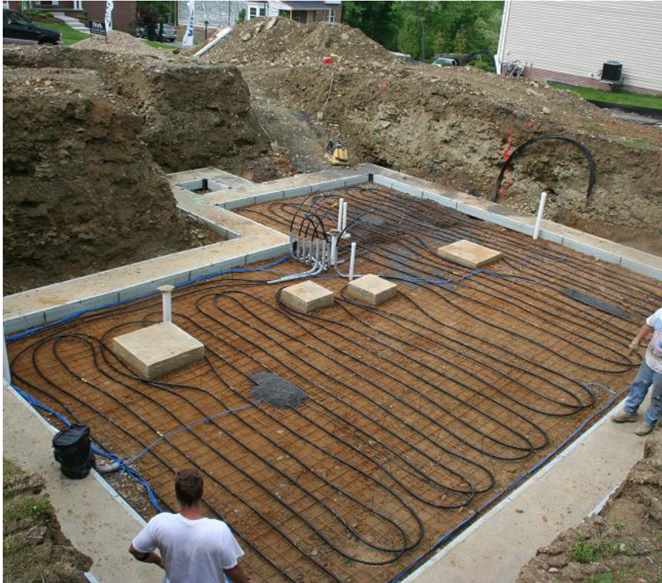
Figure 3. GSHP sub-slab ground heat exchange loop composed of \frac{3}{4} -in. high density polyethylene piping
