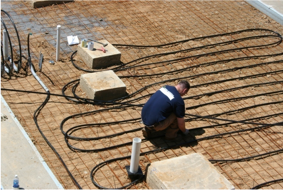
Figure 2.34: HDPE 3/4" tubing installed beneath the basement slab will serve as the ground loop for the ground-source heat pump.
