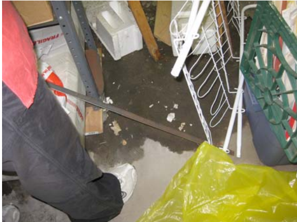
Figure 1: Damp floor in basement storage area
