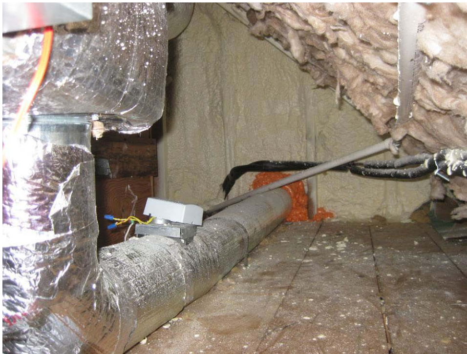
Figure 14. Millbury Cape ventilation system in kneewall
