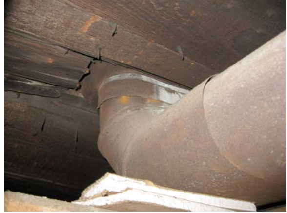
Figure 4: Supply ductwork serving 2 nd floor
