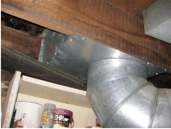
Figure 3: Panned return for 2 nd floor heating system
