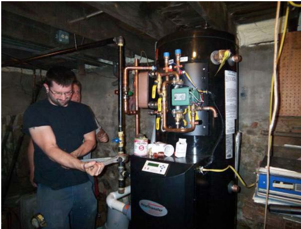
Figure 15. Somerville Triple Decker Phoenix Versa Hydro installation. Photo used with permission from homeowner.
