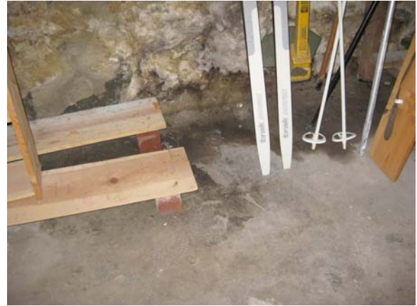
Figure 2: Damp floor and wall in basement
