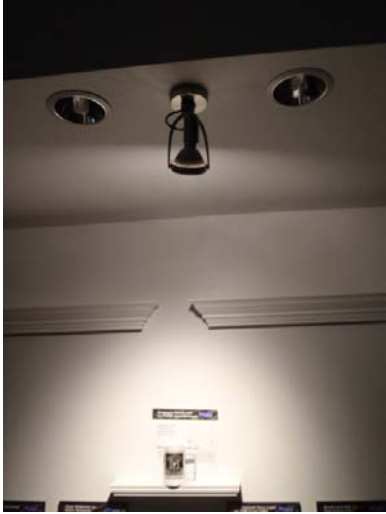
Figure 32. LED track light.
