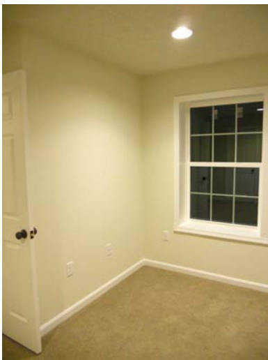
Figure 30. LED recessed downlight.
