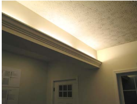
Figure 4. Architecturally integrated light cove.
