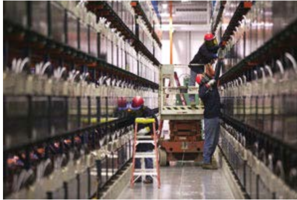
Figure C-9. Inside GVEA NiCd energy storage
