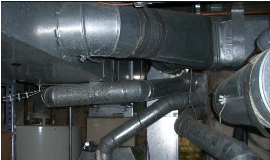
Figure 46. A tangle of metal ducts and flue pipes. Branch ducts have been sealed with duct tape which is failing (esp. in lower right). All duct seams and junctions should be sealed with mastic. Care should be taken to avoid contact with the flue piping.
