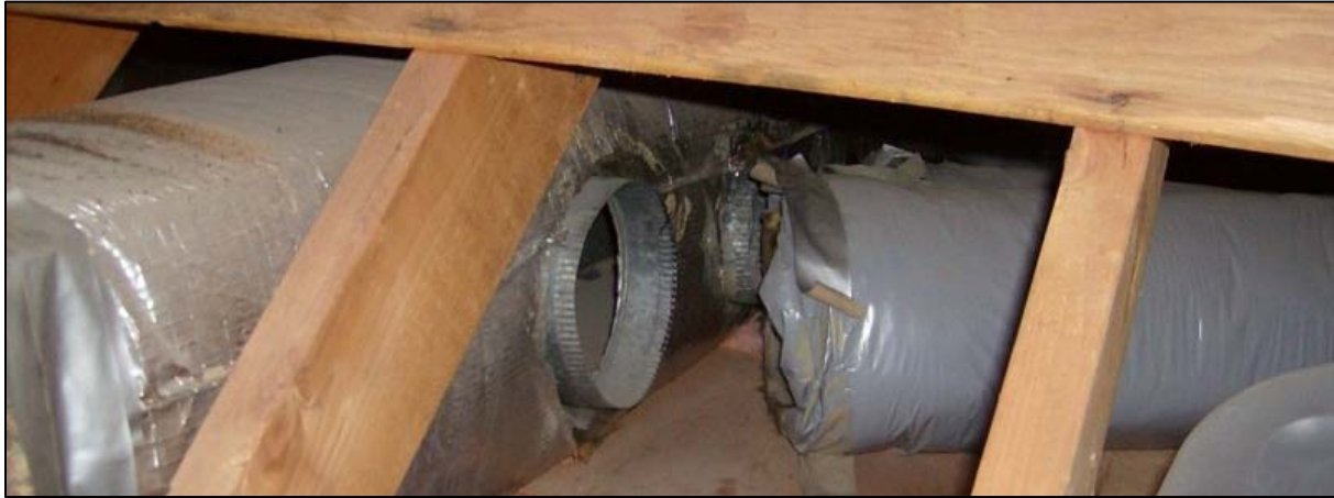
Figure 41. Disconnected ductwork resulting in conditioned air being lost to the vented attic. Homeowner was complaining of comfort issues in a secondary bedroom.
