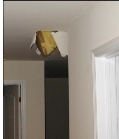
Figure 15. Ceiling damage as a result of a misplaced foot while working on ducts in an attic.
