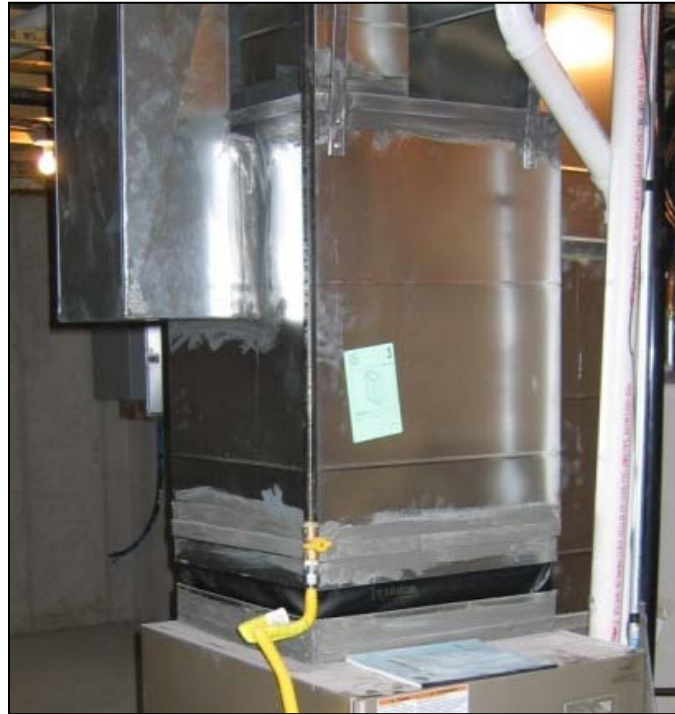
Figure 1. Sheet metal supply plenum sealed with mastic. A flexible, fireproof canvas collar was installed to provide sound/vibration attenuation.
