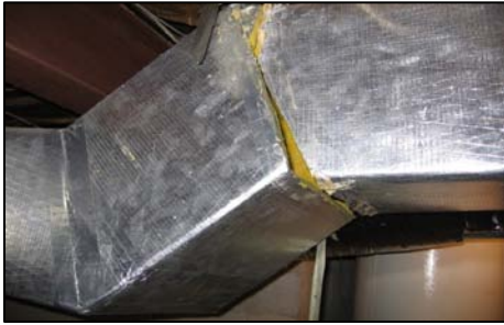
Figure 32. This duct board trunk was sealed with foil tape that has failed due to the stress put on the duct. Neither mastic nor tapes can replace proper mechanical fastening and support.
