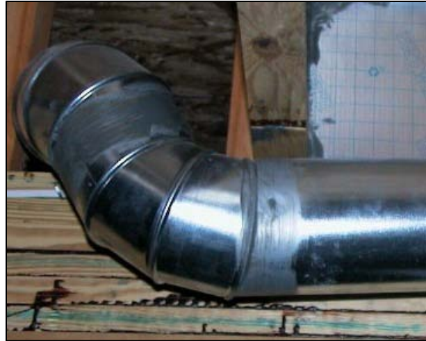
Figure 25. While sealant has been applied to some of these joints, such a thin coat may not provide an adequate seal. Follow manufacturer’s instructions for the thickness when applying mastic.
