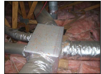
Figure 45. Duct board junction box with multiple flex branch ducts.
