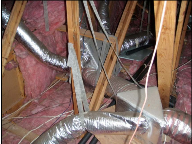
Figure 4. Insulated flex duct in the attic of an existing home
