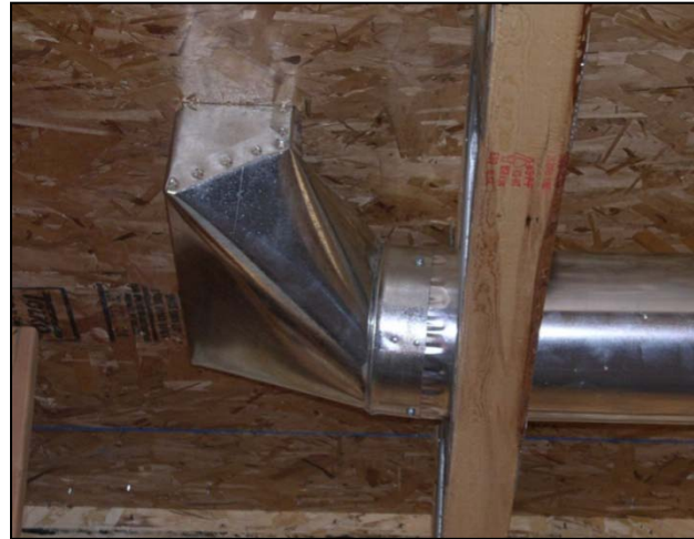
Figure 47. Sheet metal boot that has not been sealed.
