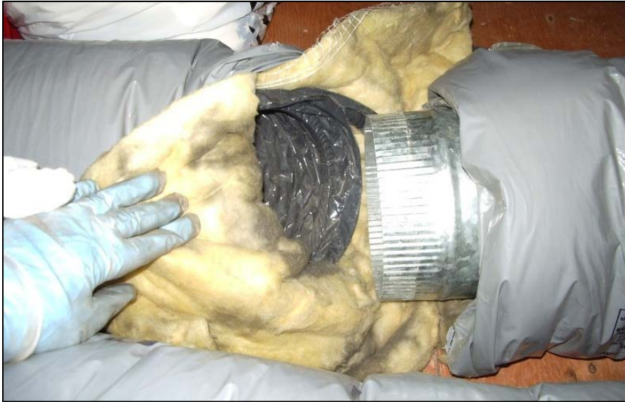
Figure 44. This flex duct junction has failed completely. The inner lining of both sections should be attached and sealed to the metal fitting. Insulation should then be taped in place.
