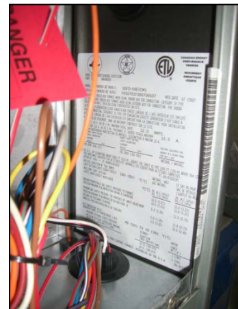
Figure 19. The specified heat rise range for this furnace is 40-70°F according to the faceplate.
