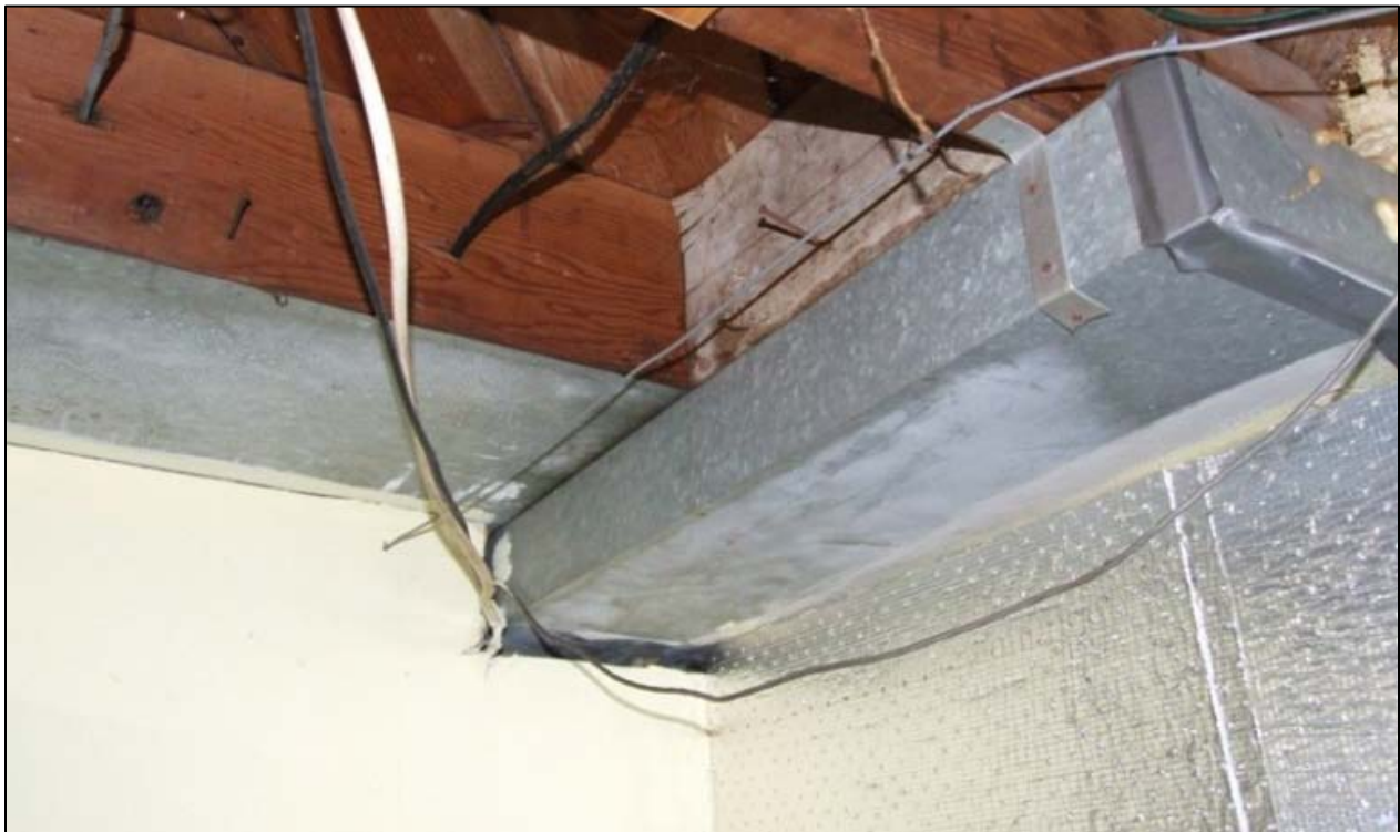
Figure 52. Hard duct, panned returns, and wood blocking are combined as part of the return system. Gaps and seams are not sealed at all, and wiring penetrations allow even more leakage.
