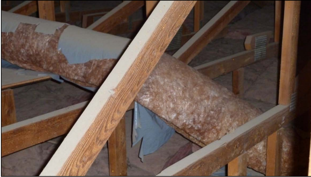
Figure 28 Vapor barrier has eroded and needs to be replaced
