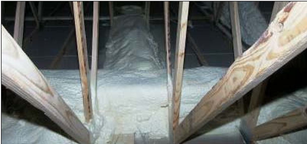
Figure 14. Ducts insulated with closed-cell spray foam in an attic. Fiberglass insulation will be blown over the ducts, providing the necessary ignition barrier.
