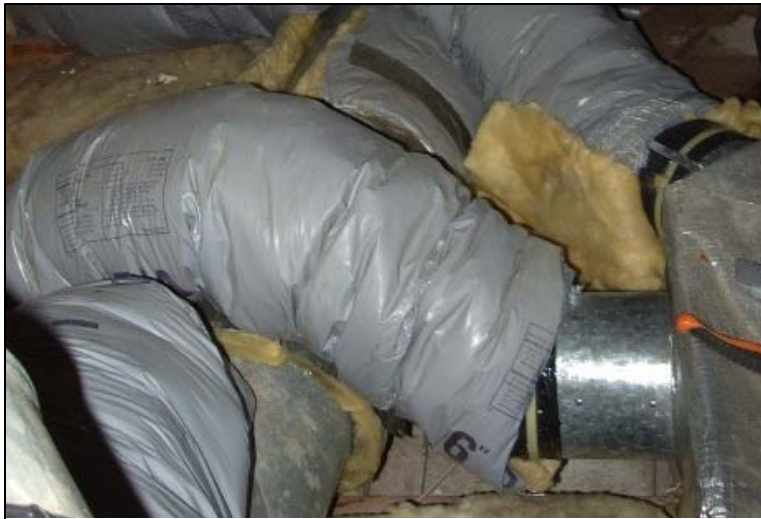
Figure 38. The inner lining of these flex duct branches have been attached to the collars, but they have not been sealed
