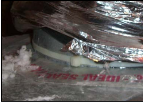
Figure 36. What exactly is being secured here?
