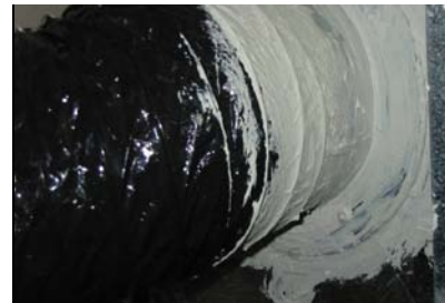
Figure 35 A flex branch (insulation pulled back) attached and sealed to a collar. Note the balancing damper; sealers must be careful that mastic does not prevent access to and operation of such devices.
