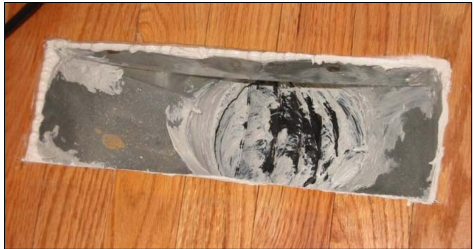
Figure 49. Mastic has been used to seal the flex duct to the register boot, seams in the sheet metal boot itself, and the gap between the boot and the floor. Sealing from the exterior is preferable, but when ducts are not accessible, this method can be utilized. As always, use proper gloves and be careful of screws and sharp edges when sealing boot connections.
