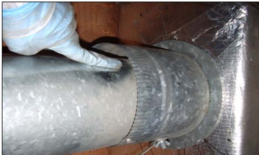
Figure 43. It appears the HVAC contractor ran out of the proper sized ducts or collars for this installation
