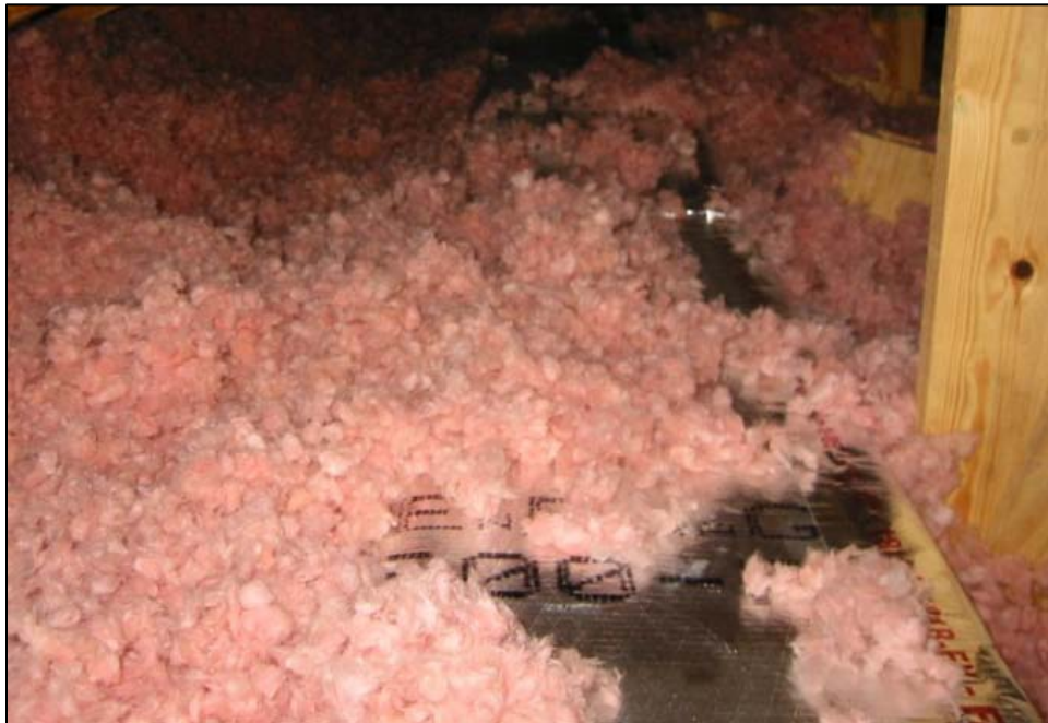
Figure 56. A duct board trunk partially buried beneath blown attic insulation. This may be impractical in existing homes and in humid climates.
