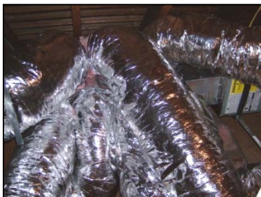
Figure 39. Having this much flex duct branching off at the supply plenum makes it very difficult to properly seal the ducts.
