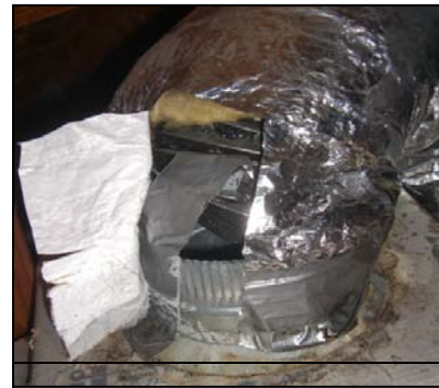
Figure 34 This flex branch never overlapped the collar and the insulation wasn't properly installed resulting in leaks and condensation.
