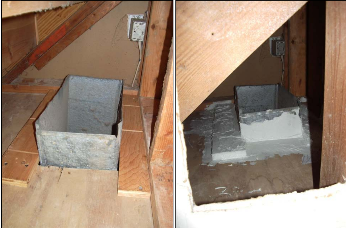
Figure 53. This space beneath a stairway was used as a return plenum. Installing a ducted return – the preferred solution – was not in the scope for this project. System performance was improved by sealing this building cavity.
