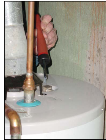
Figure 17. Spillage testing of an atmospherically vented, natural gas water heater.
