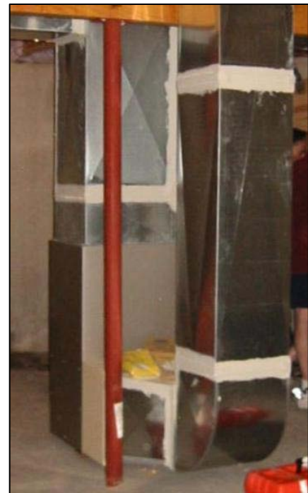
Figure 31. Supply and return plenums and trunks sealed with mastic.
