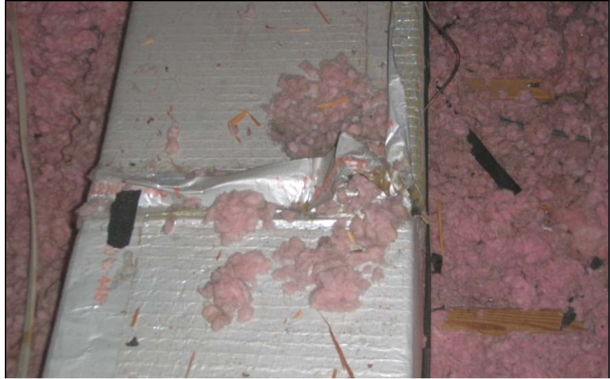
Figure 8. Aluminum tape falling off of duct board ducts.
