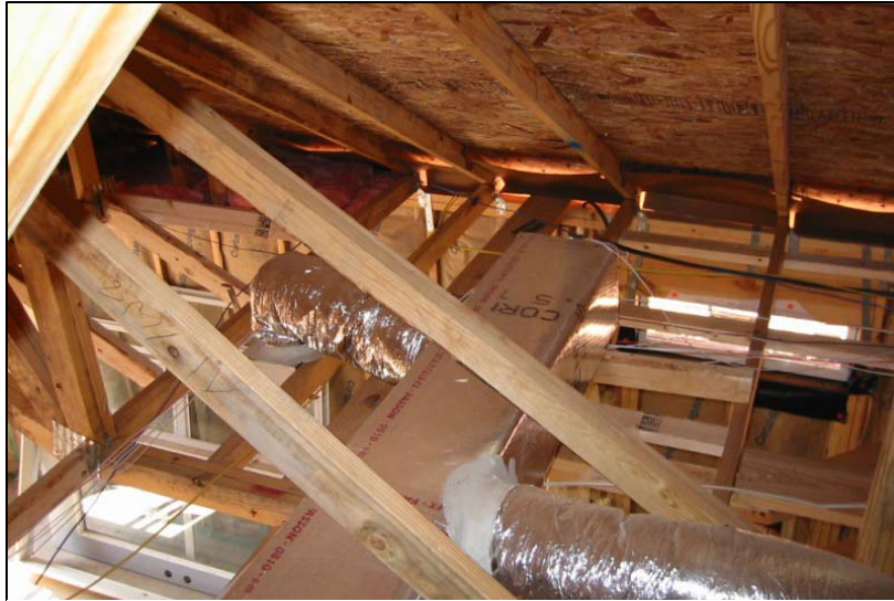
Figure 12. A duct board trunk with flex duct branches sealed with mastic.
