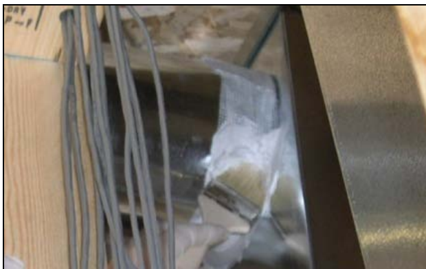
Figure 10. A duct connection being sealed using fiberglass mesh tape and mastic being applied with a paint brush.
