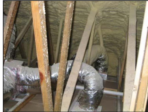
Figure 54. HVAC brought into conditioned space by applying spray foam to roof deck.
