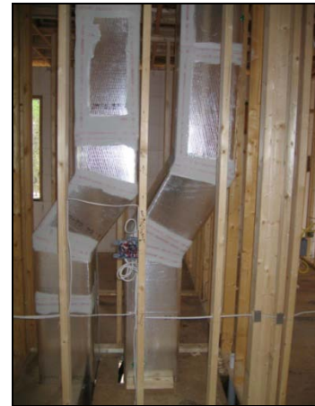
Figure 11. Duct board sealed with mastic.
