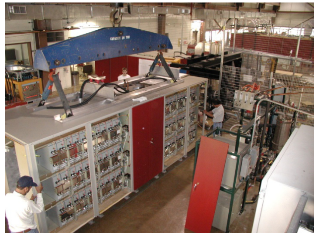
Figure 3. Completed NuMI horn power supply.
