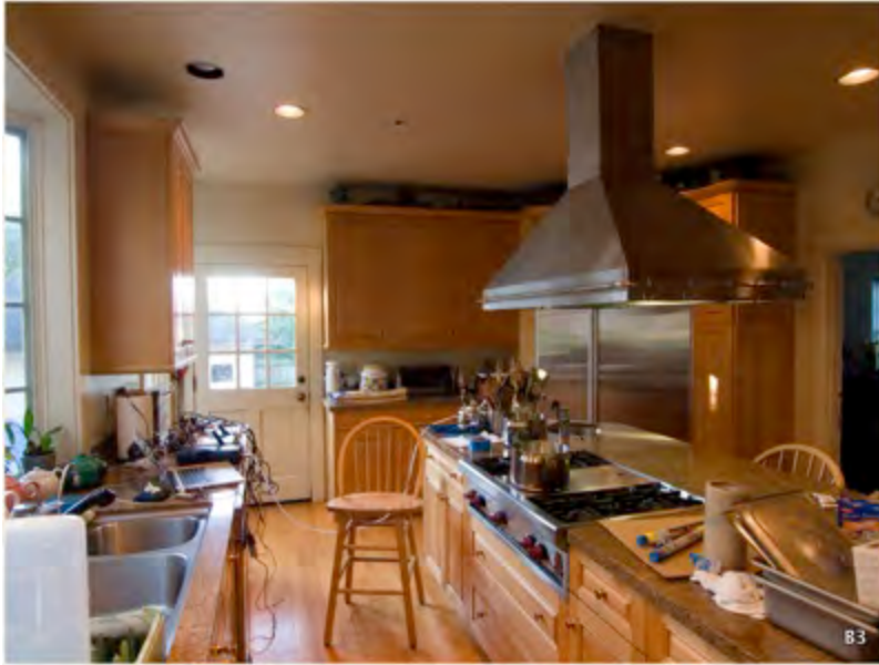
Figure 47. Exhaust System B3 showing location in kitchen.
