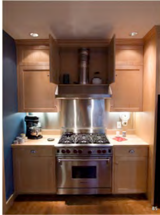
Figure 55. Exhaust System B5; placement in kitchen.
