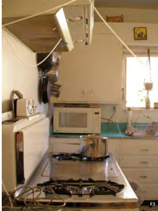
Figure 19. Exhaust system F3, side view.
