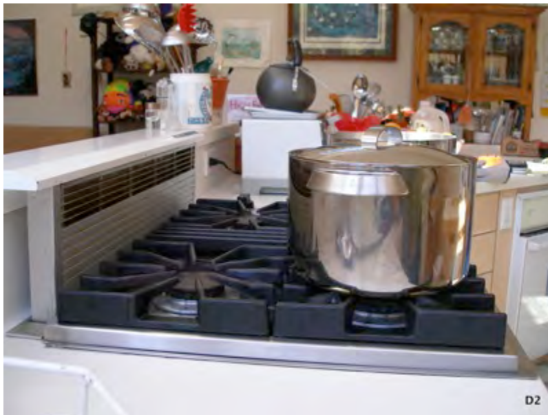
Figure 6. Downdraft exhaust system D2.
