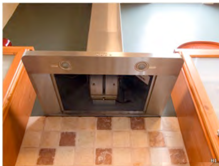
Figure 30. Exhaust System F5 with grease screens removed.
