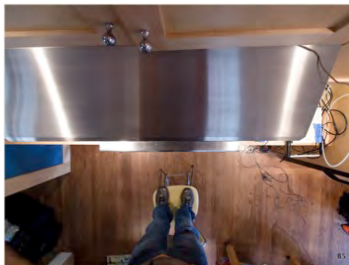
Figure 56. Exhaust System B5; top view showing coverage of cook top.
