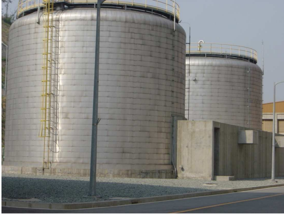
Figure 3-1 Photo of the Condensate Storage Tanks [KAERI Email Communication to BNL, 09/29/2009]
