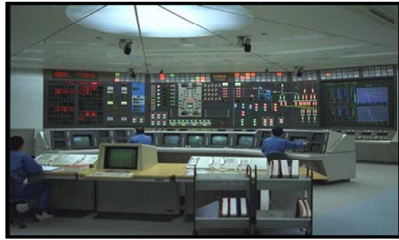
Control Room with Computer-based HSIs
