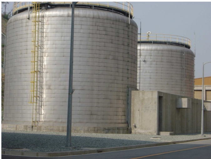
FIGURE 1 THE CONDENSATE STORAGE TANKS
