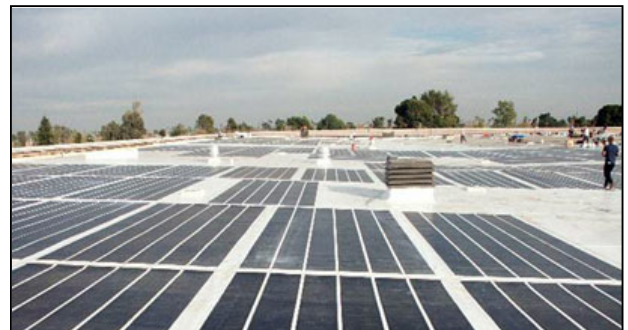
Figure E-2: Integrated PV on Base
