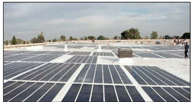
Figure E-2: Integrated PV on Base
