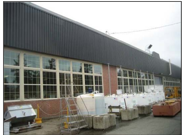
Figure E-4: Solar wall installed at Fort Lewis
