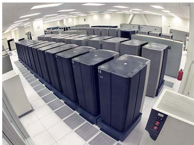
Figure 7.10. Typical Data Center
