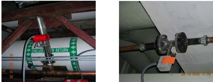
Figure 8.7. Compressed Air Meter Applications at the NIH. Meter in left photo is an insertion-type while meter in right photo is an in-line-type.
