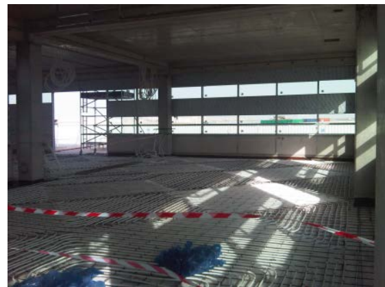
Figure 13. Masdar Institute low-lift cooling field test site progress
