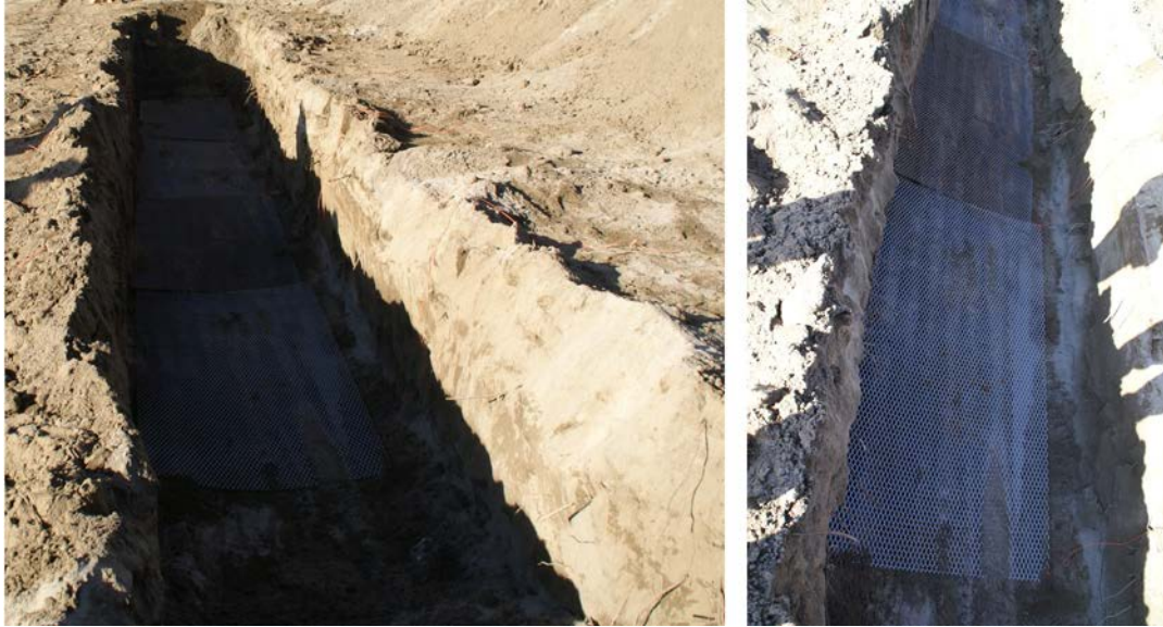
Figure 3.7. 4-ft × 32-ft Plate Buried 4-ft Deep (4 metal grates, 4 ft × 8 ft each placed end to end)
