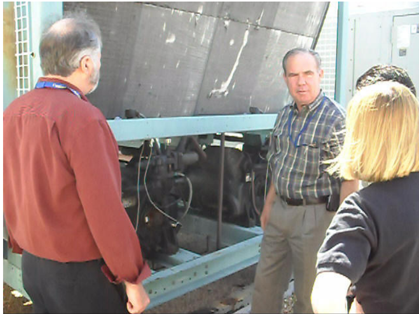
Photo 1. Jim Arends, PE, CEM, Redhorse; Charlie Watts and Dr. Pat Harrington, CBP; and Mike Savena, PE, Redhorse, inspecting RTU4 AC compressor during FEMP energy audit site visit, April 2010.
