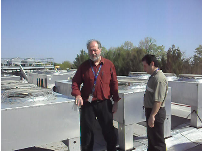
Photo 5: Jim Arends, PE, CEM, and Mike Savena, PE, Redhorse, inspecting close layout of condenser units during FEMP energy audit site visit, April 2010.
