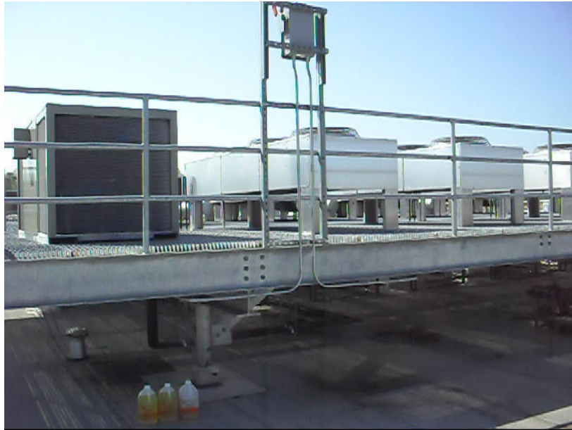
Photo 3: Condenser units on roof of data center building observed during FEMP energy audit site visit April 2010
