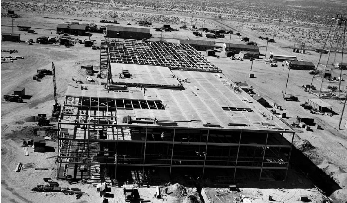
Figure A.2. 234-5Z Building Under Construction, Showing Steel Structure. Building column grid A-J (omitting I) is from right to left in this photo; column lines 1-24 begin at this eastern end and work toward the west. The 242-Z and 236-Z Buildings had not been started when this photo was taken.
