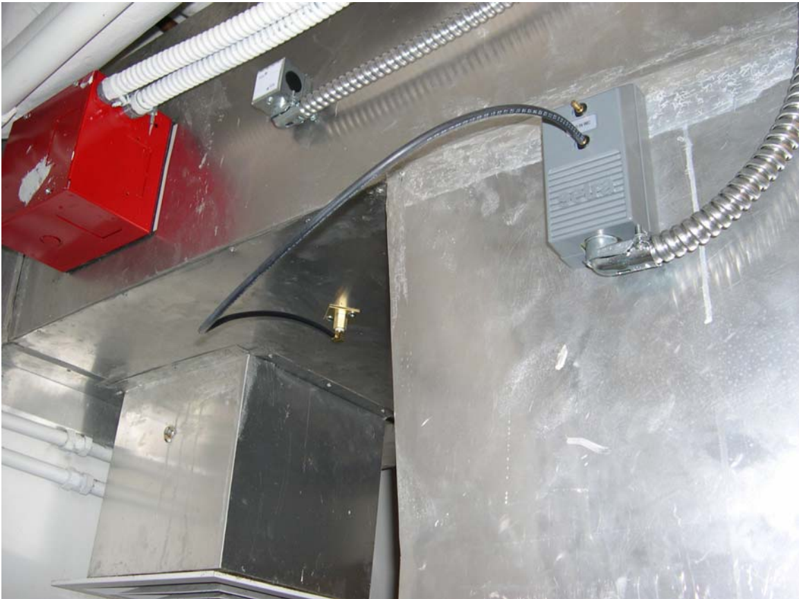
Figure 3. Sensors mounted in improper position.
