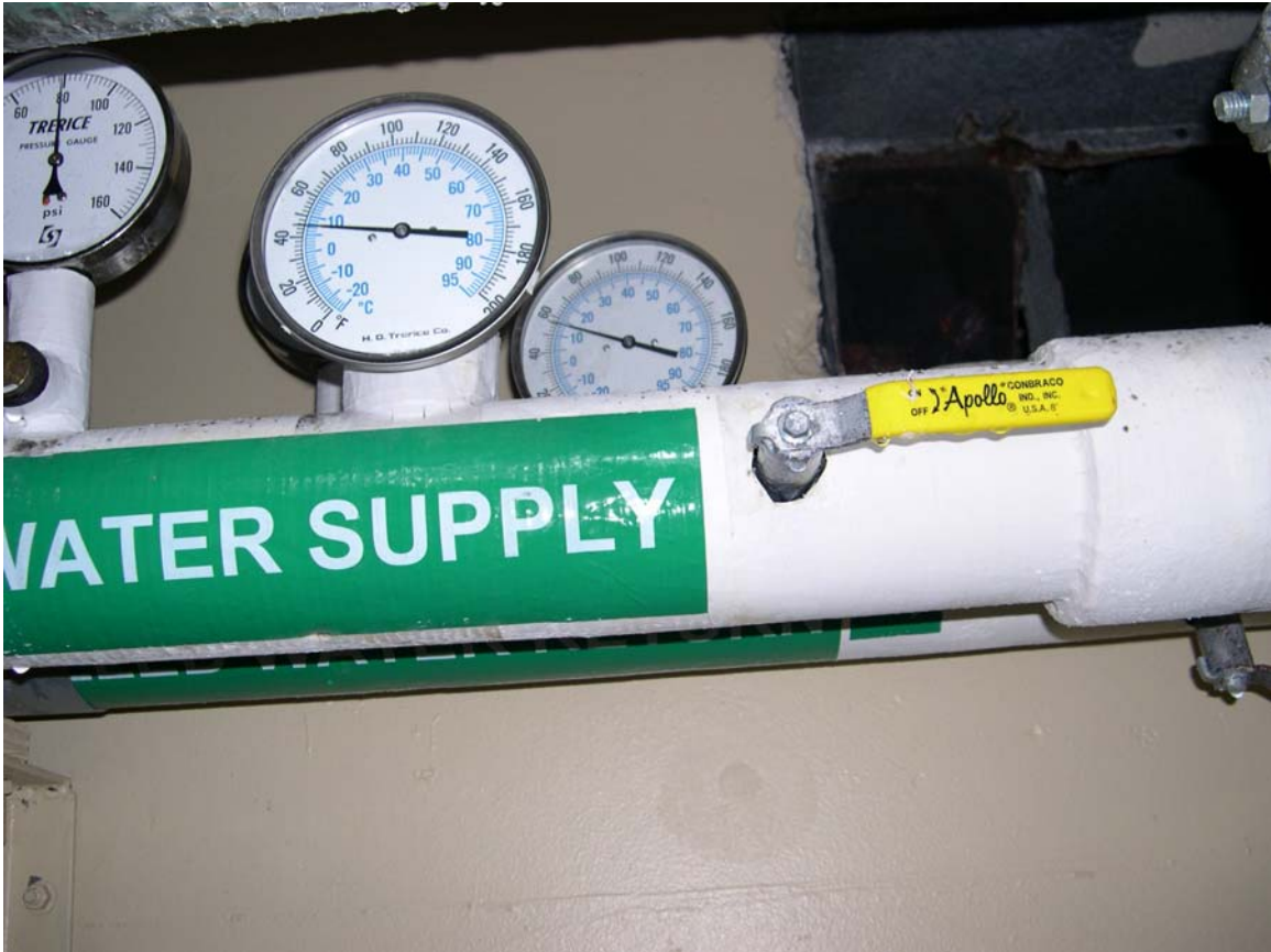
Figure 6. Chilled water supply gauges
