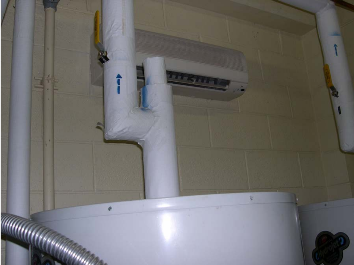
Figure 4. Split A/C unit in mechanical room
