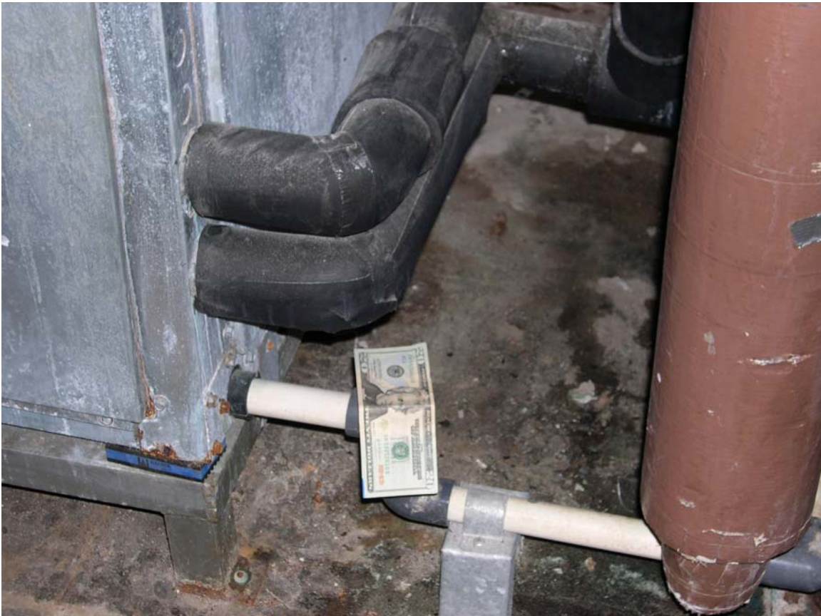
Figure 2. P-Trap line with no trap, which allows water to collect in air handler.
