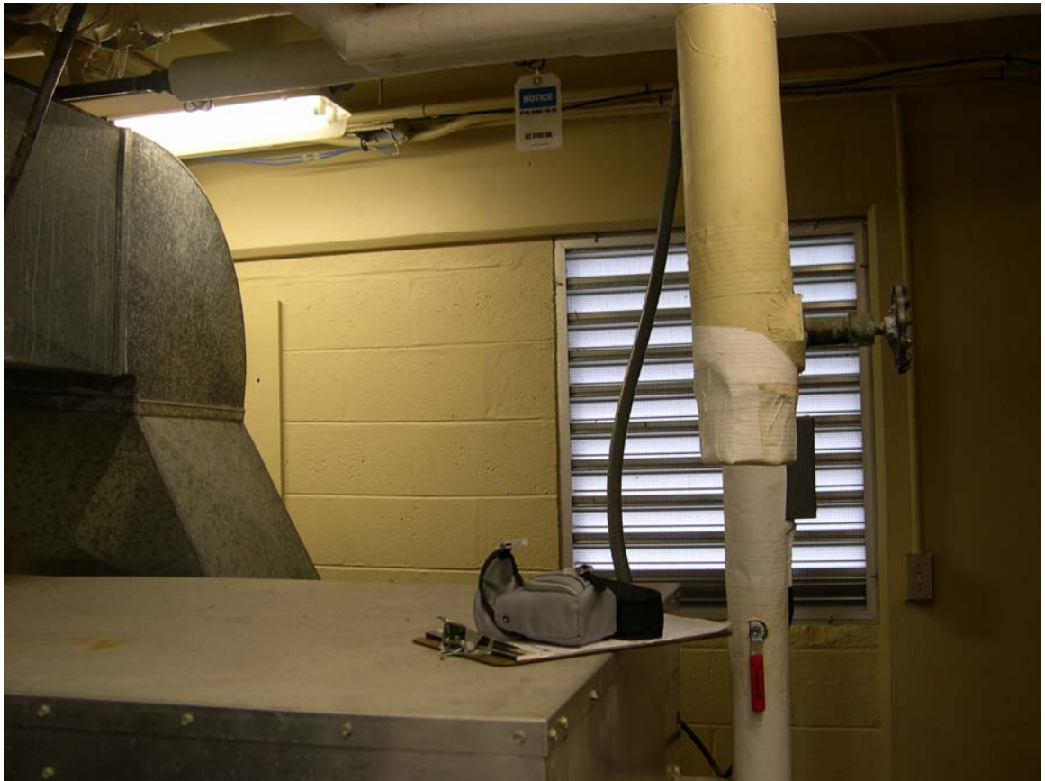
Figure 5. Fully open outside air grill.
