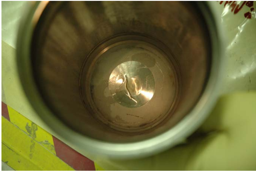
Figure 1. Moisture inside the PCV
