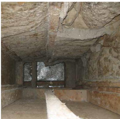
Among the home's design flaws are empty building cavities that directly connect the crawlspace and attic, creating a year-round escape path for conditioned air.
