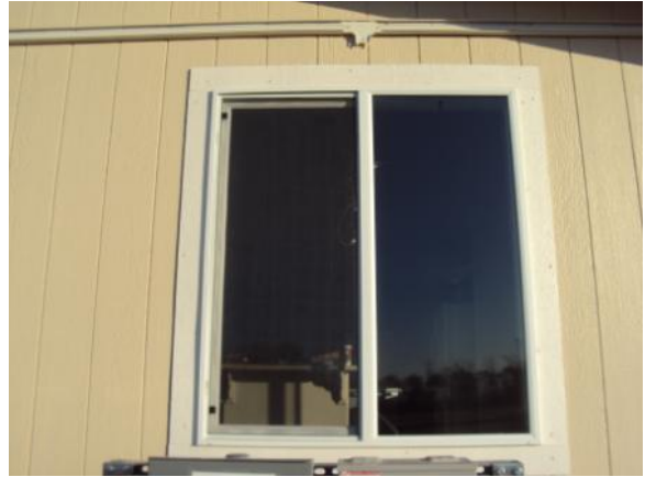
Figure 5.6. Window on West End of Experimental Home. Note conduit and “T” above window ready for thermocouple installation.
