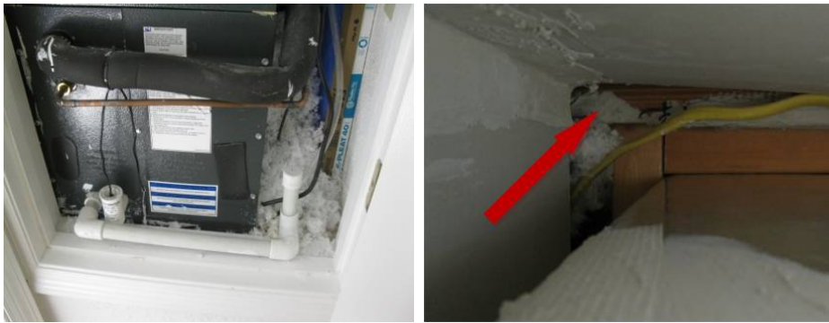
Figure K.18. Retrofit EH-07: White Attic Insulation Around Air Handler (left) Fell Through Spaces in the Closet Ceiling (right, looking up at closet ceiling framing)
