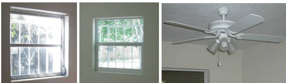
Figure K.3. Retrofit EH-02: Pre-Retrofit Awning Window (left), Post-Retrofit Low-E (center), Post-Retrofit Fan with Compact Fluorescent Lamps (right).
