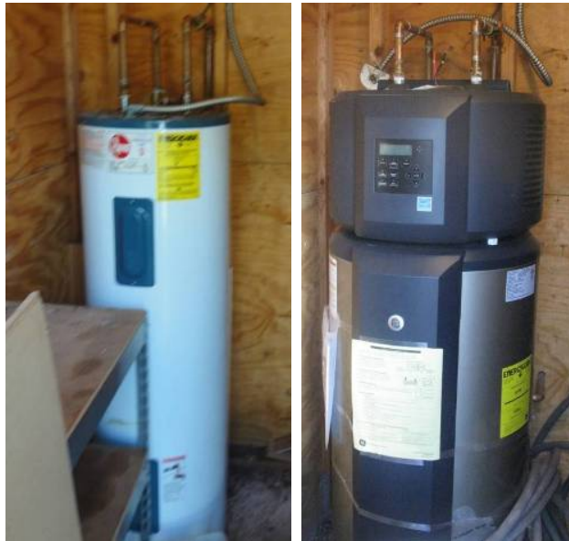
Figure K.8. Retrofit EH-03: Pre-Retrofit Electric Tank Water Heater, EF = 0.88 (left), Hybrid Heat Pump Water Heater, COP = 2.35 (right)
