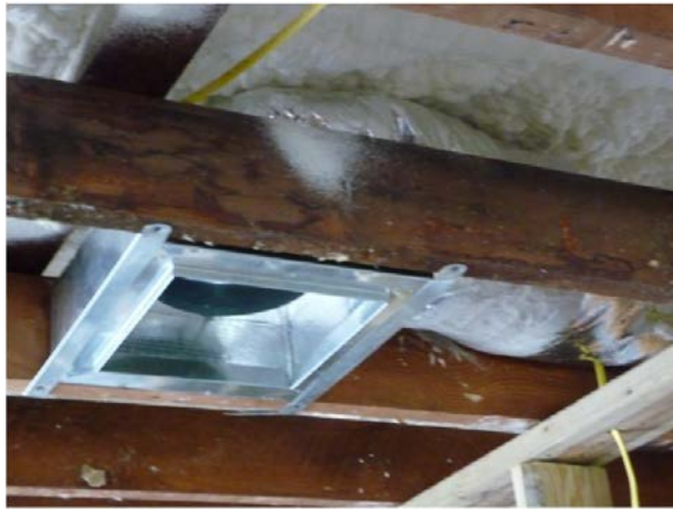
Figure K.23. Retrofit EH-14: A Very Shallow Unvented Attic with Foam Insulation at Roof Deck Resulting in Duct Compression and an Area of Thinner Insulation
