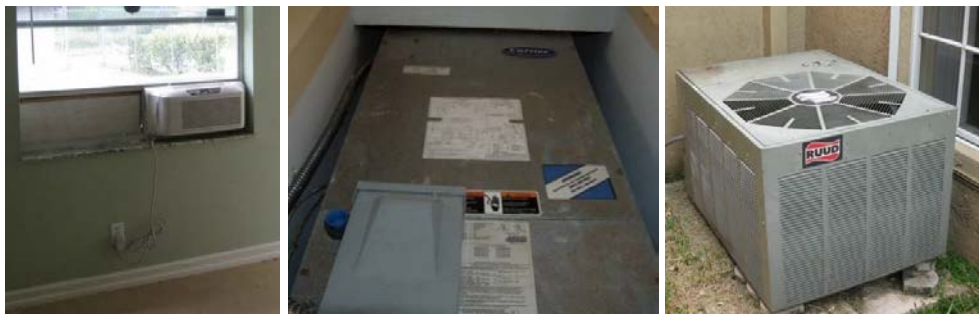
Figure K.29. Retrofit EH-21: Pre-Retrofit Wall Unit (left), Pre-Retrofit Condenser (center), and Pre-Retrofit Air Handler (right)
