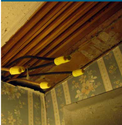
A number of holes in the ceiling allow conditioned air to escape to the attic. This gap should be covered and sealed.
