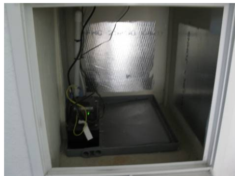
Figure K.19. Retrofit EH-07: New Return Air Plenum Constructed of Foil-Faced Duct Board, Shiny Side Facing In
