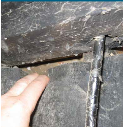
An energy analyst pulls away duct liner to reveal a gap in the return air pathway. The gap allows warm air to escape the house in winter and hot air to enter in summer. This is a common problem when builders use framed building cavities as return air ducts instead of installing metal ductwork.
