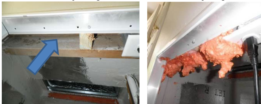
Figure K.12. An Open Wall Cavity Connecting the Return Plenum to the Attic Was Discovered During the Test-Out (left photo with arrow marking air pathway). The opening was sealed using a combination of fiberglass (filler) and expandable foam sealant/insulation (photo right). The excess foam was trimmed before reinstalling the air handler filter and grille.
