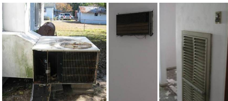
Figure K.2. Retrofit EH-02: Pre-Retrofit Package Unit (left), Wall Unit (center), Abandoned Furnace (right)
