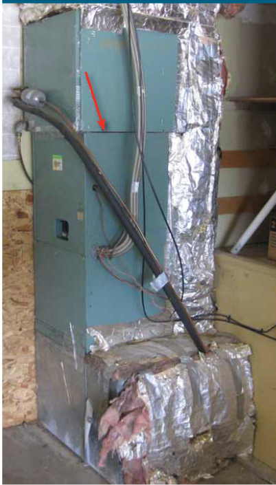
The sections of the air handler are so poorly fitted that air rushes out through gaps.
