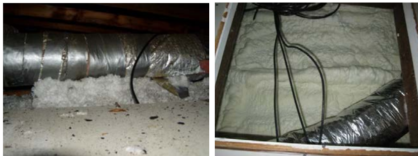
Figure K.22. Old Duct Work with Blown-In Ceiling Insulation Pre-Retrofit (left photo) and Looking Up at Insulated Roof Deck with New Ductwork Inspected Prior to Hanging Sheetrock Ceiling (right photo)
