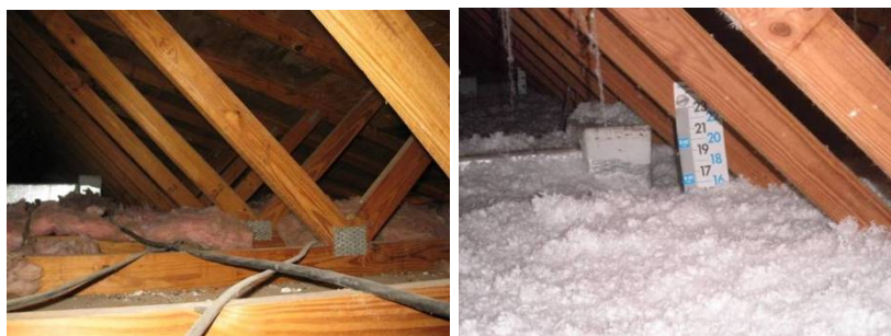
Figure K.13. Pre-Retrofit Compressed Fiberglass Insulation (left) Was Improved to R-38 with Blown-in Fiberglass
