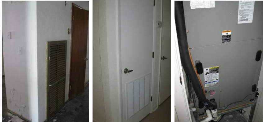
Figure K.4. Retrofit EH-02: Pre-Retrofit Abandoned Heater (left), Post-Retrofit Closet (center), and Post-Retrofit Open Return with Airflow-Restricted Louvered Doors (right)
