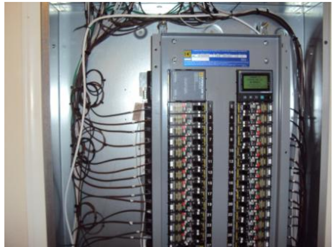
Figure 5.10. Close-Up of the Electrical Panel. Note the manually programmable interface (top right) to control the breakers and the loops on the conductor wire to increase measurement accuracy.
