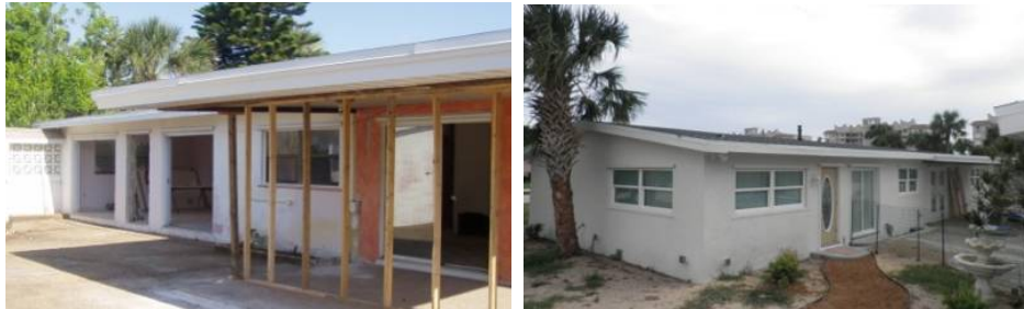
Figure K.20. EH-14 Pre-Retrofit with Deconstruction Already in Progress (left) and Post-Retrofit (right)
