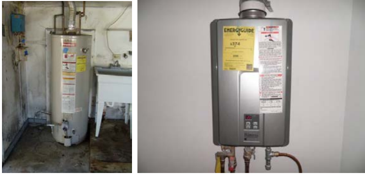
Figure K.21. Externally and Internally Located Water Tanks. Switching from an exterior located gas hot water tank (left photo) to an interior mounted instantaneous tank (right photo) reduced the HERS index by 7 points and saved an estimated $491/yr. in energy use.
