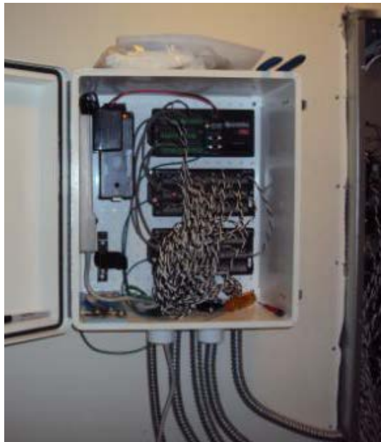
Figure 5.11. The Campbell Scientific Data Logger and Termination Panels Used to Measure Electrical Power via Circuit Transducers
