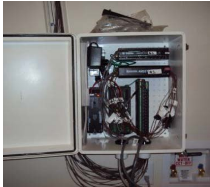
Figure 5.12. The Second Data Logger Used to Measure Temperature, Humidity, and Other Parameters as Well as Control Functions.
