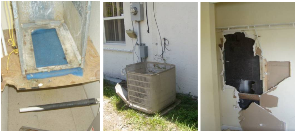
Figure K.25. Retrofit EH-19: Pre-Retrofit Air Handler (left), Compressor (center), and Interior Wall Destruction (right)
