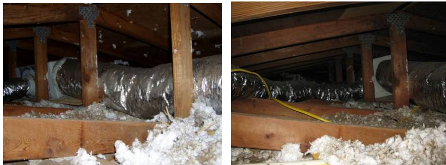
Figure K.16. Retrofit EH-06: Ceiling Insulation Pre-Retrofit Estimated Average of R-11 (left) and Post-Retrofit No Additional Insulation (right)
