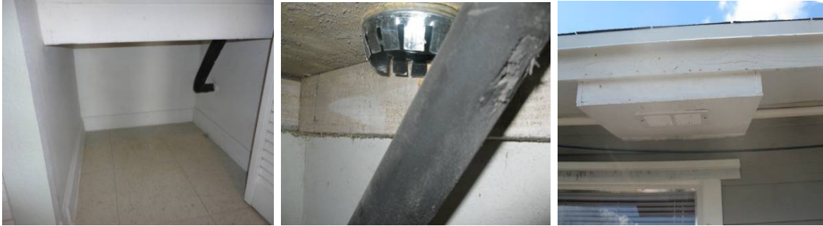
Figure K.7. Retrofit EH-03: Pre-Retrofit Return Plenum (left), Outside Air Ducted into the Post-Retrofit Return Plenum (middle), and Soffit Retrofit for the Air Intake (right)
