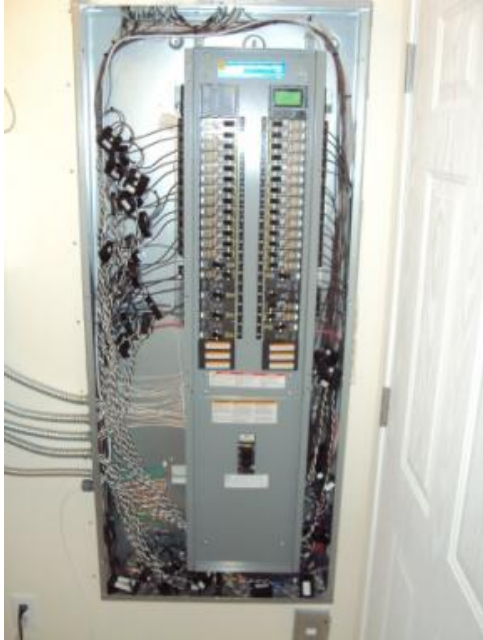
Figure 5.9. Fully Instrumented Electrical Panel with Current Transformers on All 42 Circuits
