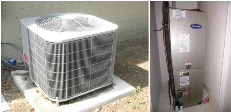
Figure K.11. Replacing the SEER 9 Air Conditioner and Gas Furnace with a SEER 13 Heat Pump Accounted for the Greatest Reduction in Estimated Annual Energy Cost ($277) of Any Single Measure in this Project.
