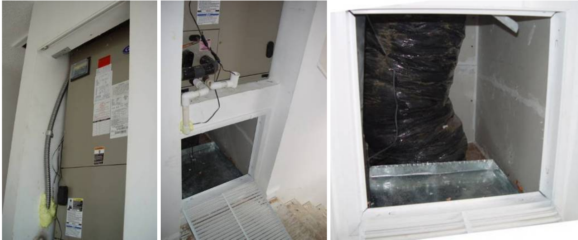
Figure K.31. Retrofit EH-21: Post-Retrofit Air Handler Closet (left), Post-Retrofit Closet (center), and Post-Retrofit Open Return with Airflow-Restricted Louvered Doors (right)
