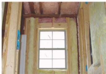
Insulation was well installed in this project without gaps or compression (Photo sources – BSAG and Calcs-Plus)
