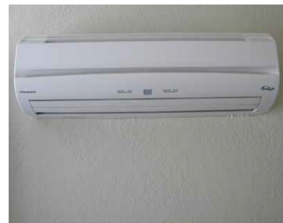
The home has never had a heating system. Building America researchers recommend installing a ductless, mini-split heat pump that will bring a year-round improvement in comfort. Wall-mounted units like this one will provide heating and cooling.
