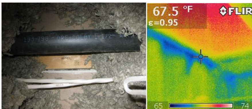
Figure 2. Left: Attic air leak. This is the top plate of an interior wall as seen from the attic. As you can see, there is crack between the top plate and the sheetrock that allows air to move between the attic and interior walls. The crack is small, but it runs the entire length of every interior wall. Right: This is an infrared image of a 2 nd floor interior wall. Colder air from the attic is moving down into the walls. Air leaks in the attic can be sealed with caulk or spray foam (again, fire-rated materials must be used where appropriate).
