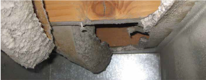
The home's builder avoided installing a metal duct for return air by using this building cavity instead. Worn fiberglass batt insulation can be seen in this close-up of the building cavity. Fiberglass inside a duct may pose a health hazard. Minute shards of glass can be pulled into the airstream and circulated around the house.
