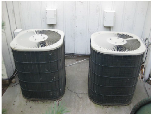
Above: Two air conditioning units which are original to the house and about 14 years old with a SEER 10.
