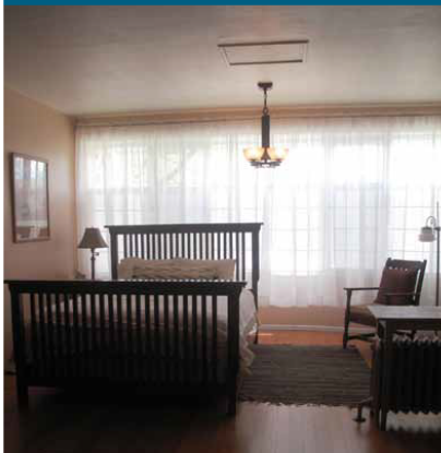
In the master bedroom, breezes stir the curtains even when the leaky casement windows are closed. The uninsulated floor is also chilly; it extends over the open front porch.
