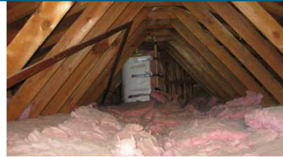
The Building America researchers recommend adding insulation to the attic at either the floor or ceiling level. This will yield only minor savings but will increase comfort in the rooms below.
