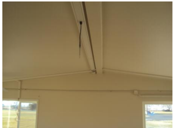
Figure 5.8. Conduit Running Parallel to the House Marriage Line. Interior RH sensor is attached to the conduit.
