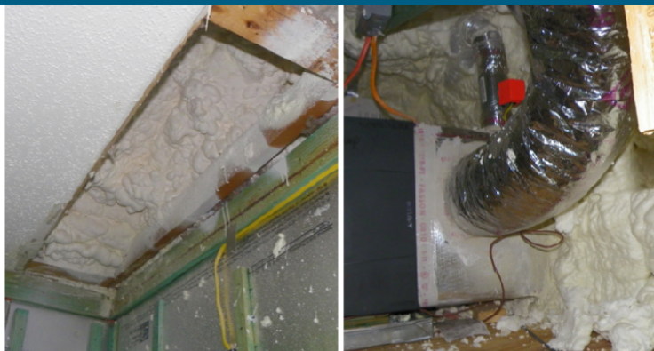
Ceiling drywall was removed along the perimeters of the home to access the attic. Open-cell spray foam was sprayed along the underside of the low-pitch roof to provide an R-21 air sealed, insulated attic space to house the new SEER 16.25 heat pump. (Photo Sources: Calcs-Plus)
