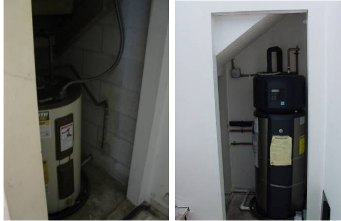
Figure K.30. Retrofit EH-21: Pre-Retrofit Electric Tank Water Heater (left) and Post-Retrofit Electric Hybrid Water Heater with Heat Pump (right)
