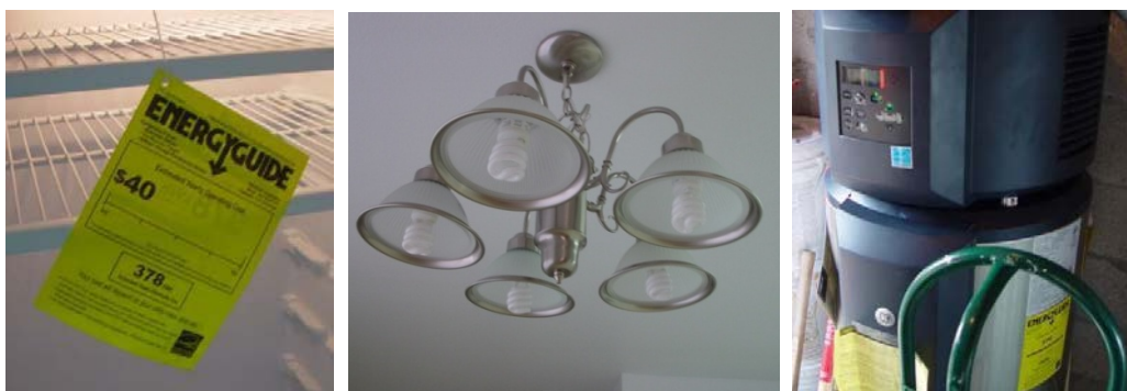
Figure K.26. Retrofit EH-19: Post-Retrofit ENERGY STAR Refrigerator (left), CFL Fixture (center), and Heat Pump Water Heater
