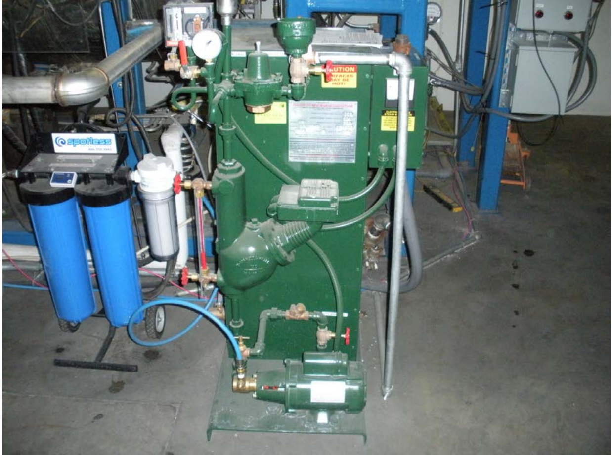
Figure A.11. Gasifier Boiler
