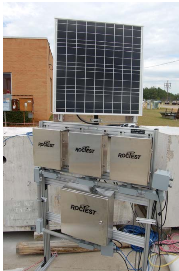
Figure 3-5. Structural frame built to hold multiplexer, data logger and solar panel and controller units
