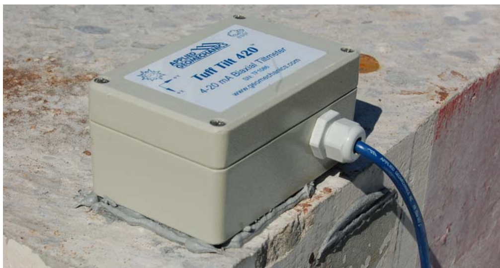
Figure 3-7. Tiltmeter mounted to the top of a block
