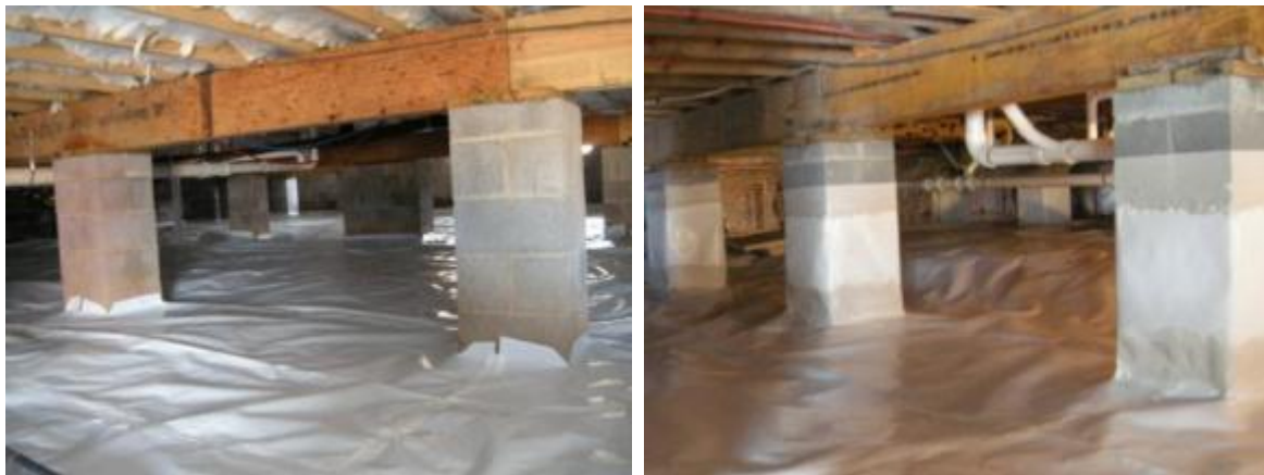
Figure 4. Vented crawlspace in WC3 (left); walls insulated and sealed in WC4 crawlspace (right). Notice that there are no ducts in either crawlspace.
