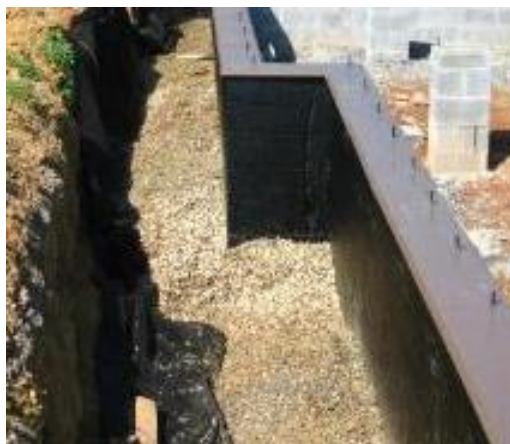
Figure 3. Tremco waterproofing on the exterior of the concrete masonry unit (CMU) crawlspace wall.
