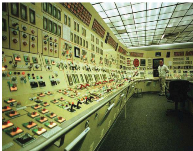
Figure 3-5. A contemporary control room at a nuclear power plant.
