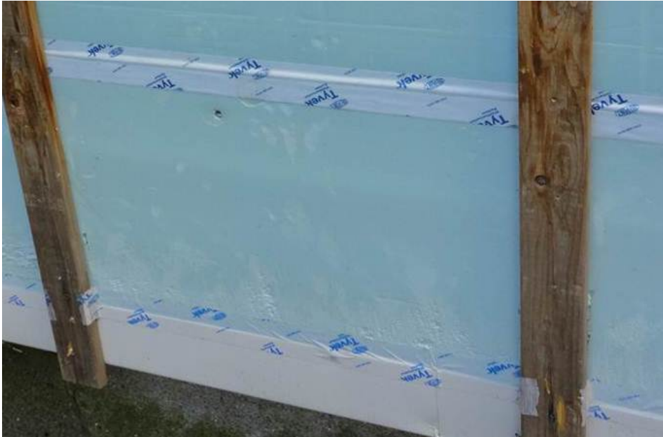
Figure 7. Exterior insulation tape inspected following 16 years of service
