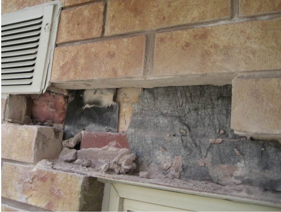
Figure 3. Intrusive investigation of the water management details. Note the poor execution of the mechanical penetration, the gap in sheathing membrane continuity, which will allow water and air leakage, and the bonding of the mortar to the membrane.
