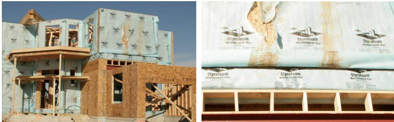
Figure 12. Examples of construction issues with traditional sheathing membranes
