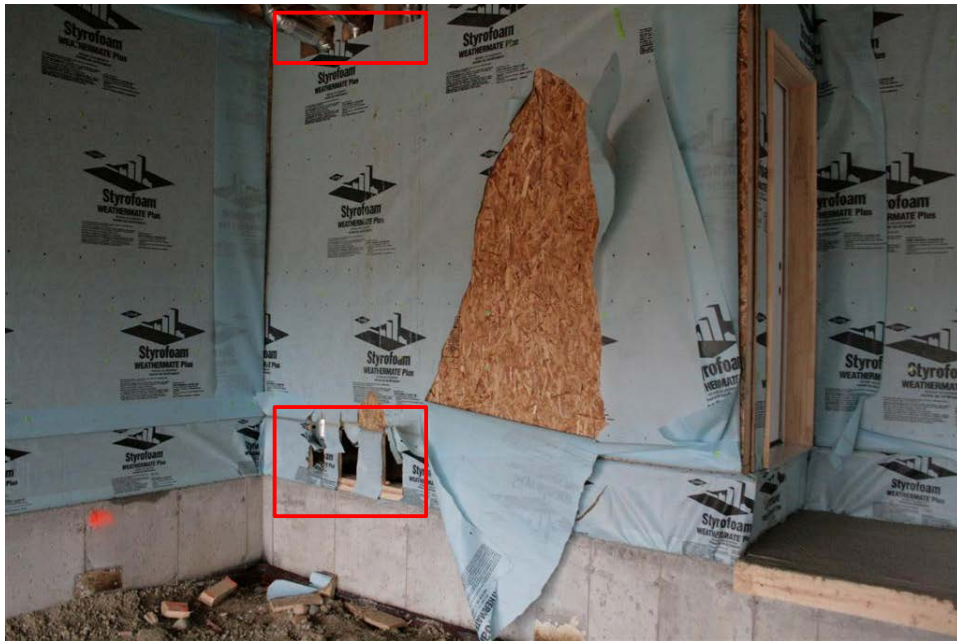
Figure 1. House wrap installation in new construction. The large tear will likely be fixed before construction continues — see one manufacturer’s instructions in Figure 2. The smaller deficiencies (highlighted) are often not addressed.
