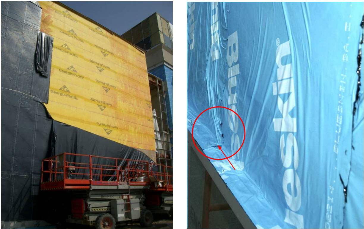
Figure 5. Self-adhered membrane installation issues
