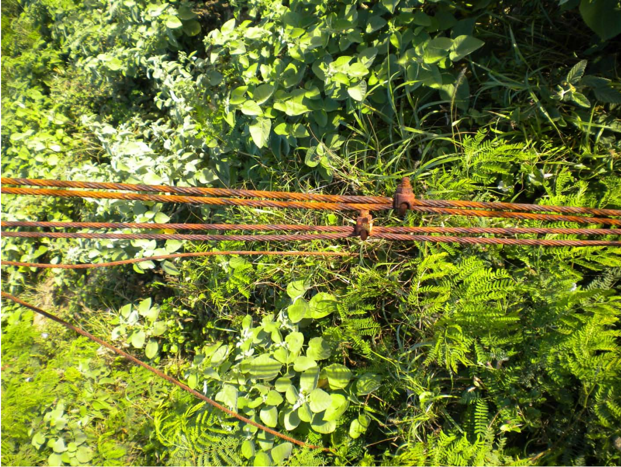
Figure 34. Guy wire degradation due to marine effects at MCBH Kaneohe Bay.
