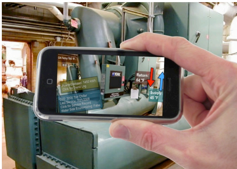
Figure 68. Mockup of augmented reality use case for chiller diagnostic (Source: NREL)
