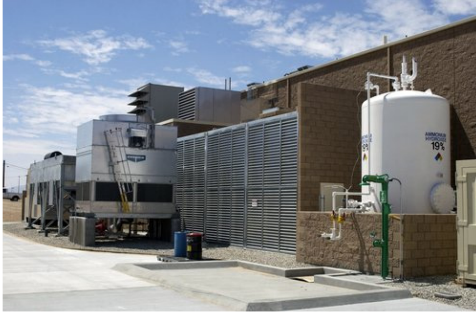
Figure 37. A 7-MW cogeneration system is part of a comprehensive set of energy and facility upgrades at a Marine base in Twentynine Palms, California (Source: NREL PIX 12709)
