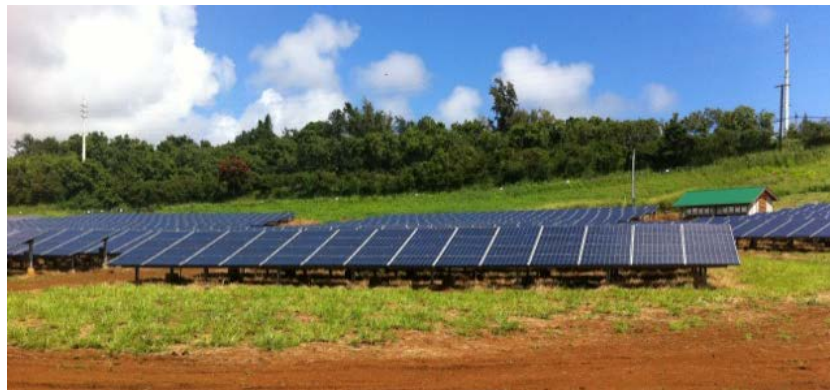
Figure 4-1. 1.2 MW Photovoltaic array on Kaua'i, HI
