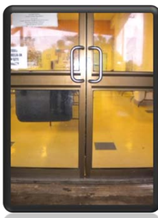
Figure 29. Visible gaps in door at Dededo Senior Center Source: NREL/PIX 18584
