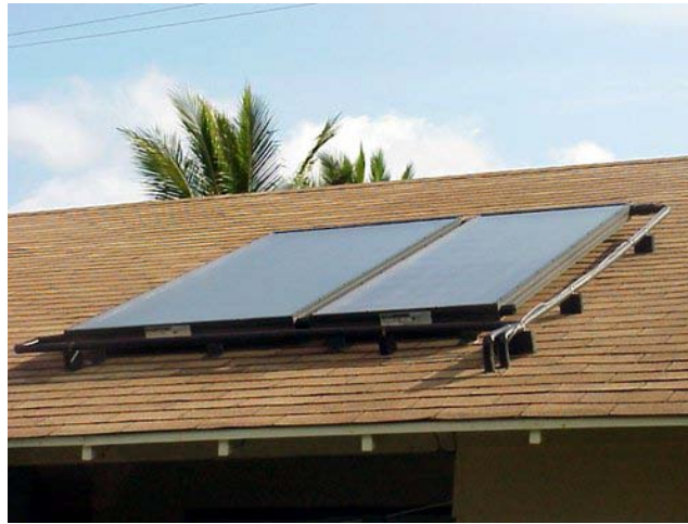
Figure 21. Solar hot water, Hickam Air Force Base Source: NREL/PIX 09188
