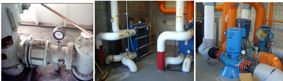
Figure 2. District Heating System Photos
