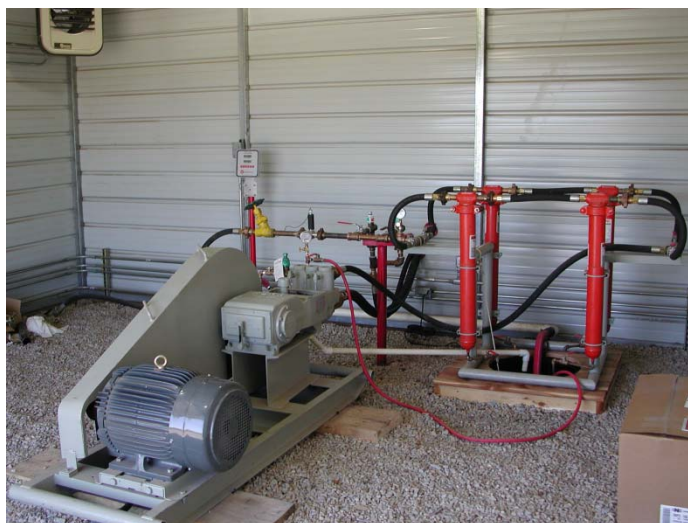
Figure 5.2.3: CO2 Pilot water injection pump and filters.
