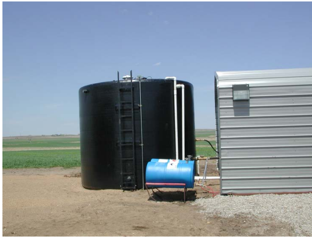
Figure 5.2.2: CO2 pilot water injection tanks and tank battery. with treatment chemicals.
