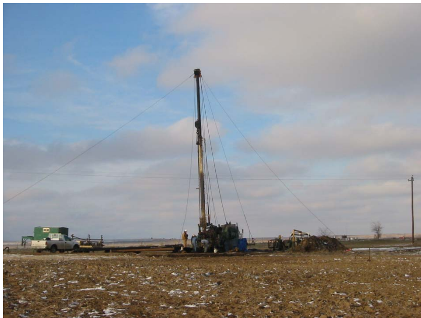
Figure 5.1.5: Workover rig on the CO 2 Project #10 water injection containment well in early March 2003.
