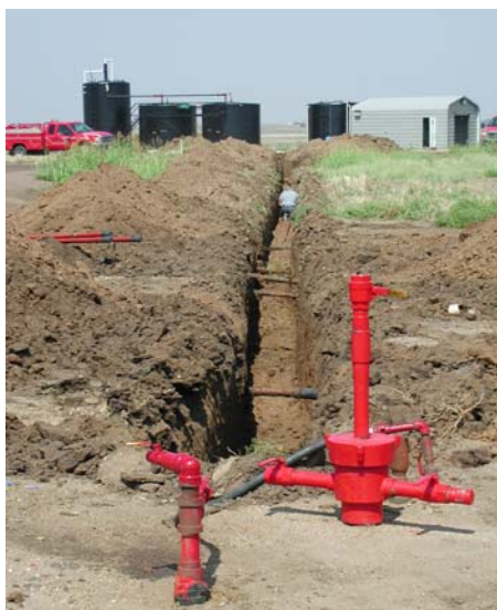
Figure 5.2.4: Laying fiberglass injection line from the water supply plant to the CO2#10 water injection containment well. View is looking to the northwest.
