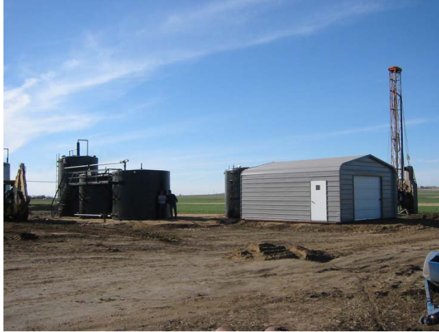
Figure 5.2.1: CO2 Injection plant near CO2 Project Injection Tanks and Tank Battery
