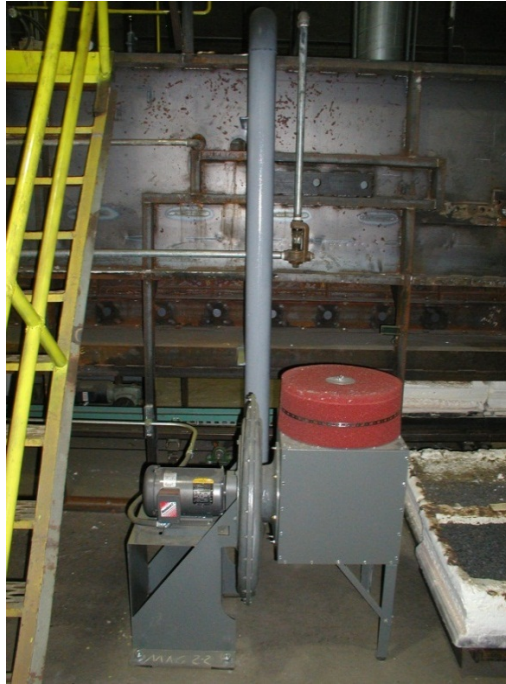
Figure 4-18. Blower for Conveying Coal
