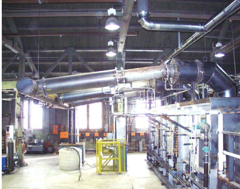
Figure 4-3. Linear Hearth Furnace Exhaust Ductwork
