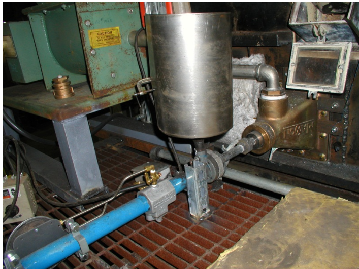
Figure 4-17. Oxy-coal Burner, Orifice Plate and Eductor System
