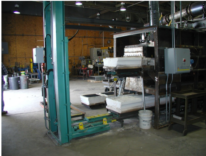
Figure 4-16. Furnace Moving Car System – Discharge
