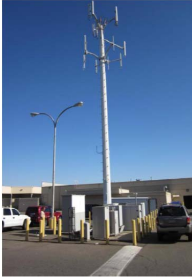
Figure 22. Photograph of a cell phone tower.
