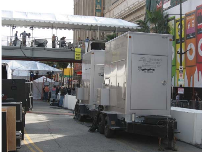
Figure 20. Two paralleled towable studio generators (300 kW, 2500A Movie Quiet each) in use at the 2011 Oscars by Saunders Electric. Note the space restrictions that can occur at such deployments. Photo courtesy of Saunders Electric.
