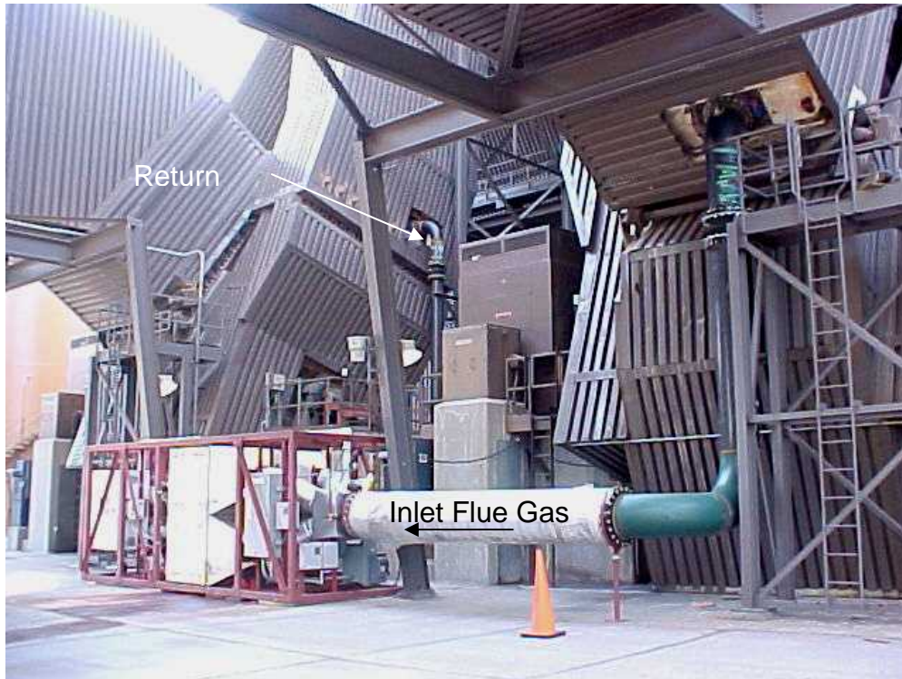
Figure 2. Pilot Oxidation Catalyst Skid as Installed at Coal Creek Station
