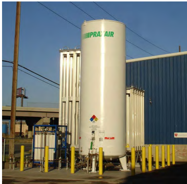
Figure 17. Praxair O 2 tank (capacity: 6,000 gallon)
