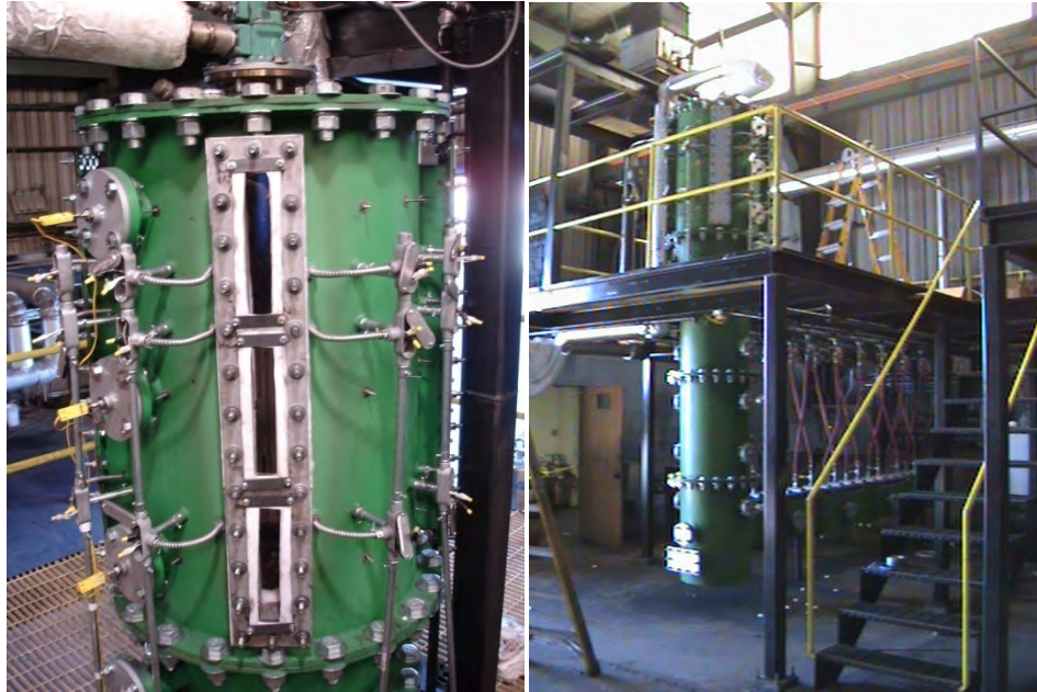
Figure 6. OFC constructed in University of Utah. Left: top section when burning NG; Right: a whole view
