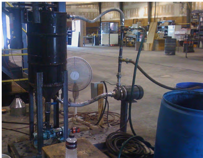
Figure 47. Prototype coal slurry feed system. The progressive cavity pump body is seen below the tank, the motor for the mixer is vertically mounted in the upper-left corner of the photo. The recirculation pump is near the center of the photo.
