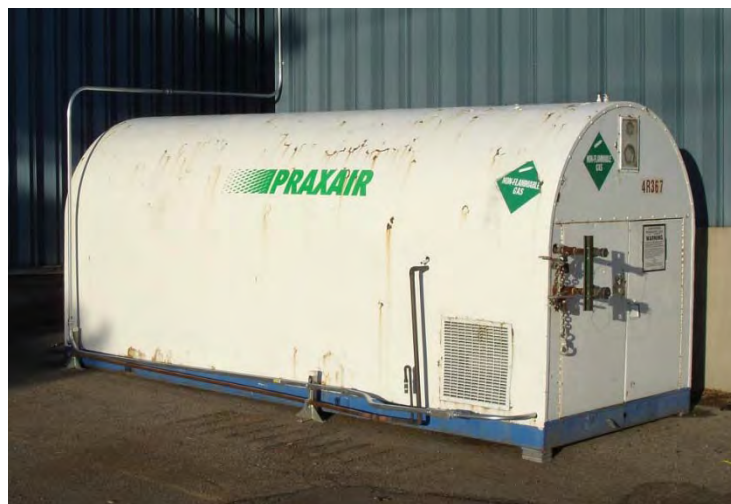
Figure 18. Praxair CO 2 tank 3 (capacity: 400 gallon)
