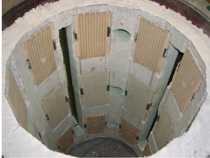
Figure 4. View of inside of top section chamber, showing electric heaters and view of optical windows
