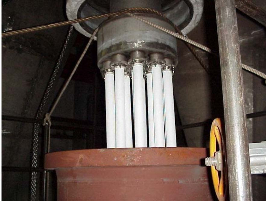
Figure 2: Image of filters mounted in slipstream vessel
