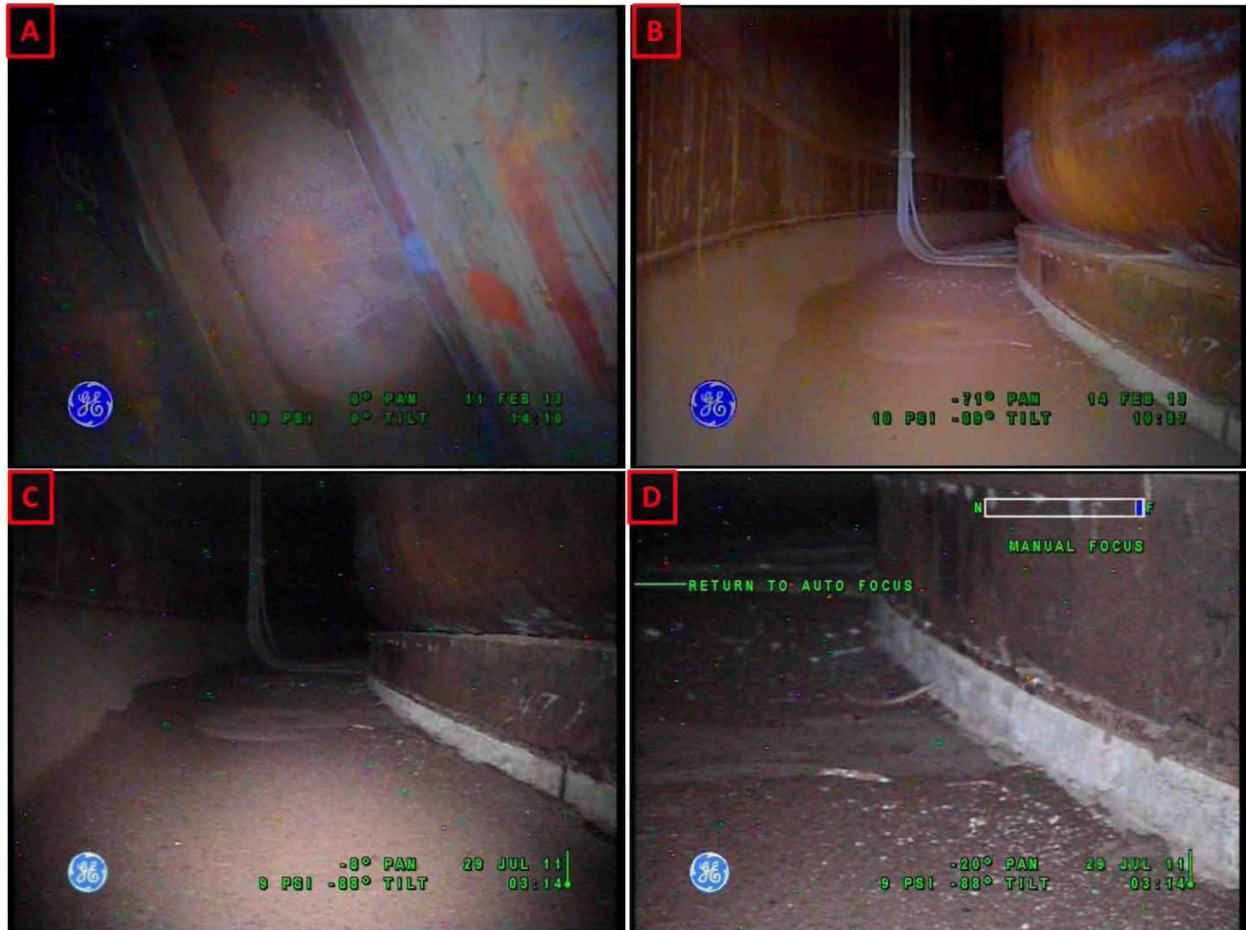
Figure 4-2. Annulus Floor Discoloration in Tank AZ-102 as seen from Riser 92 in 2013 (A), from Riser 80 in 2013 (B), from Riser 80 in 2011 (C), and Close Up View Showing Elevation Differences as seen from Riser 80 in 2011 (D)
