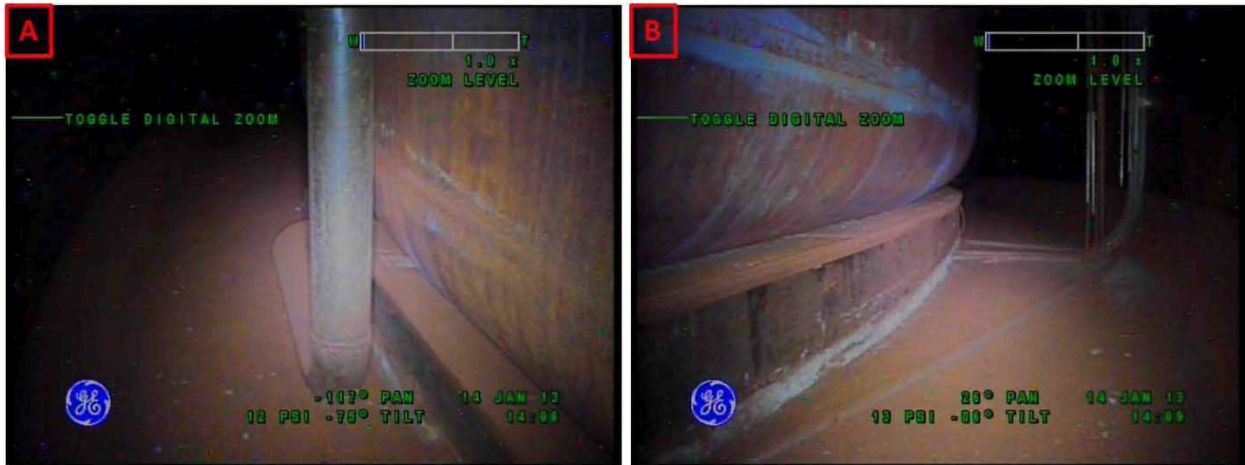
Figure 2-8. Riser 79 Lower Knuckle and Annulus Floor Condition on January 14, 2013 Looking Towards Riser 80 (A) and Looking Towards Riser 99 (B)
