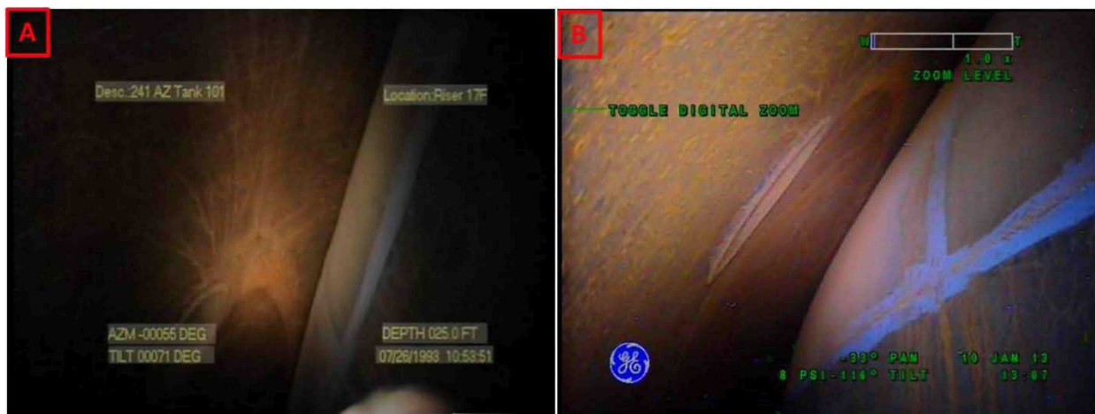
Figure 2-18. Riser 83 Upper Haunch Comparisons Between Inspections on July 26, 1993 (A) and January 10, 2013 (B) Looking Towards Riser 96
