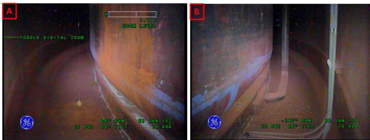
Figure 2-32. Riser 88 Lower Knuckle and Annulus Floor Condition on January 9, 2013 Looking Towards Riser 90 (A) and Looking Towards Riser 104 (B)
