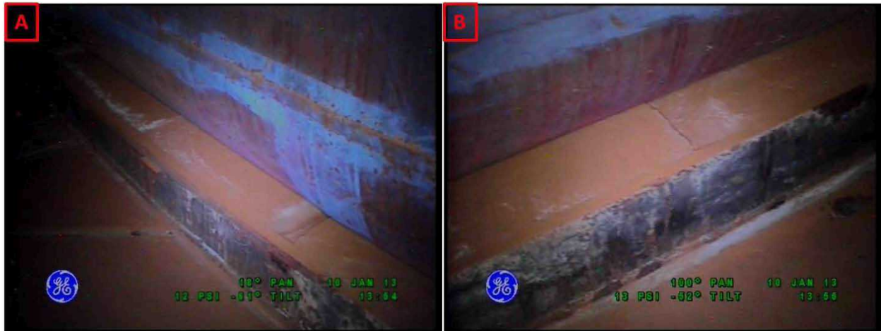
Figure 2-22. Riser 83 General Condition of the Refractory Slots on January 10, 2013
