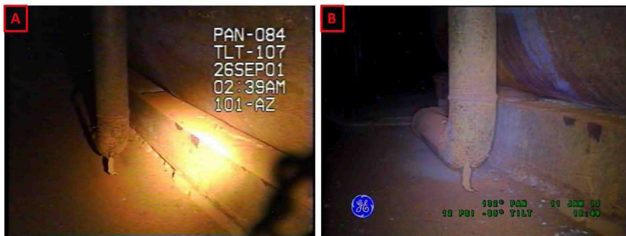
Figure 2-15. Riser 82 Lower Knuckle and Annulus Floor Comparisons Between Inspections on September 26, 2001 (A) and January 11, 2013 (B) Looking Towards Riser 95
