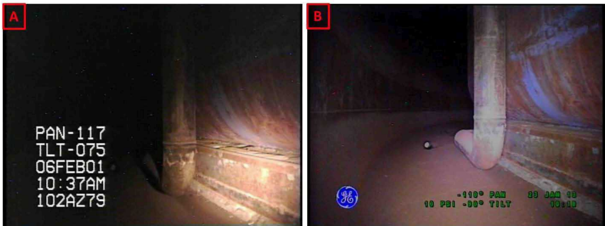
Figure 3-7. Riser 79 Lower Knuckle and Annulus Floor Comparisons Between Inspections on February 6, 2001 (A) and January 23, 2013 (B) Looking Towards Riser 80
