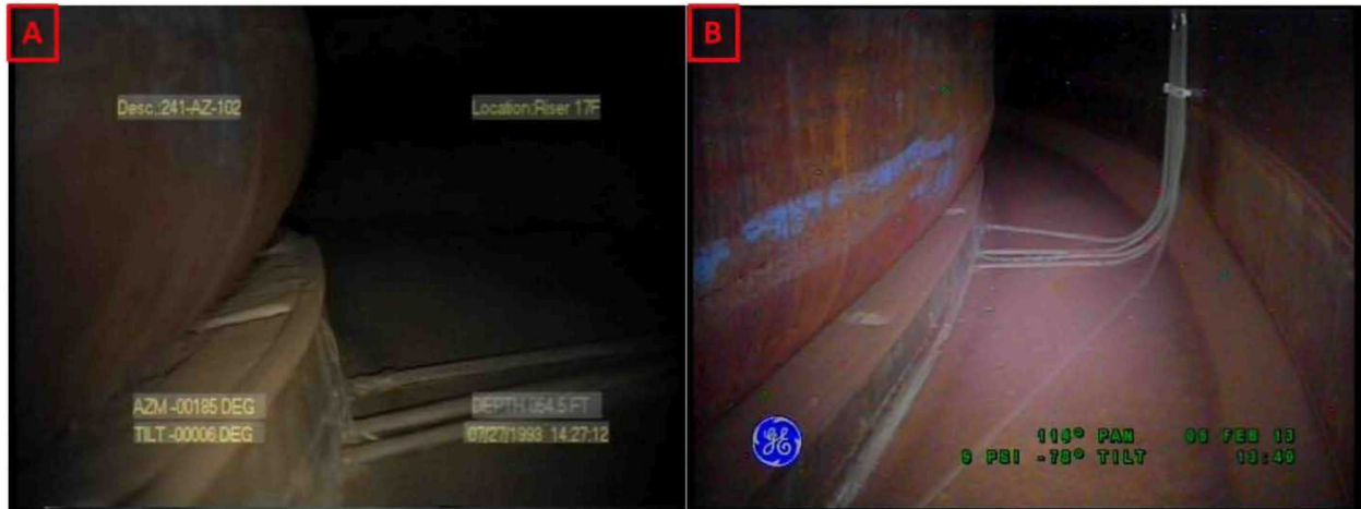
Figure 3-27. Riser 84 Lower Knuckle and Annulus Floor Comparisons Between Inspections on July 27, 1993 (A) and February 5, 2013 (B) Looking Towards Riser 102
