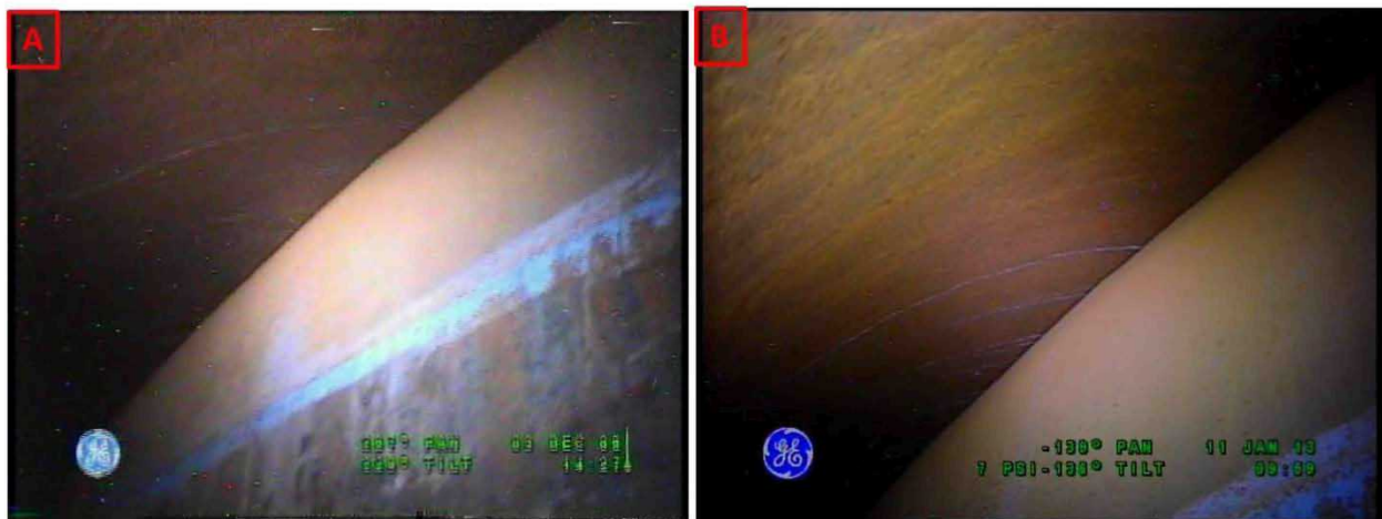
Figure 2-13. Riser 82 Upper Haunch Comparisons Between Inspections on December 3, 2008 (A) and January 11, 2013 (B) Looking Towards Riser 95
