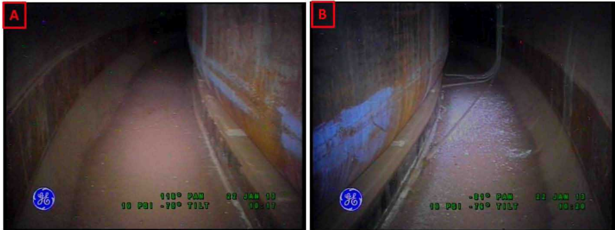
Figure 3-16. Riser 81 Lower Knuckle and Annulus Floor Condition on January 22, 2013 Looking Towards Riser 105 (A) and Looking Towards Riser 100 (B)
