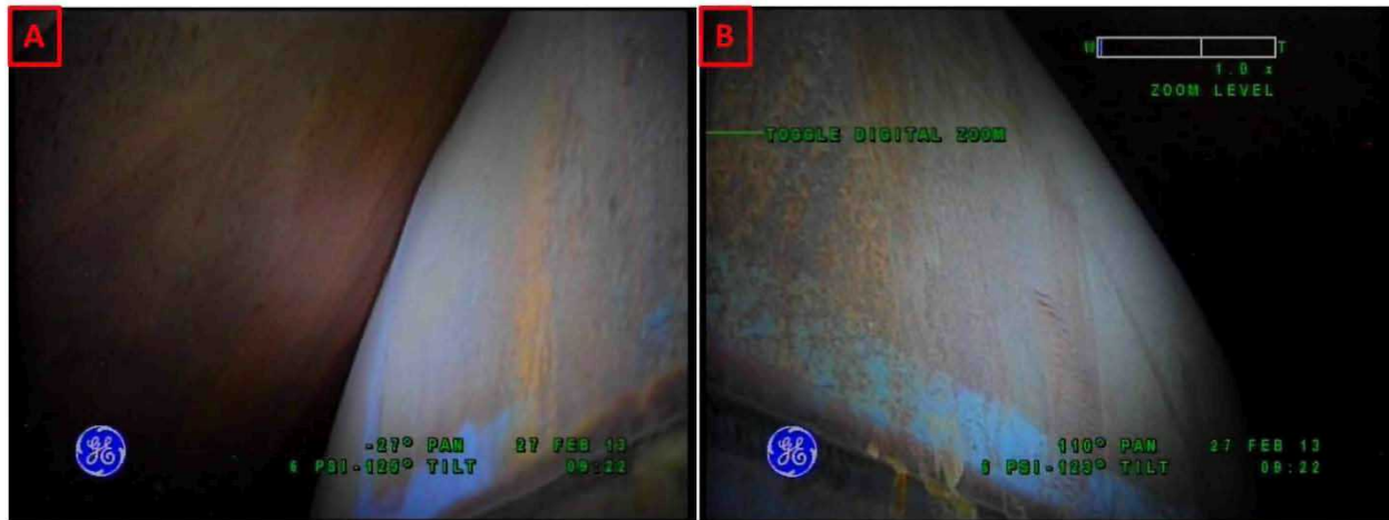
Figure 3-35. Riser 89 General Condition of the Upper Haunch on February 27, 2013 Looking Towards Riser 83 (A) and Looking Towards Riser 101 (B)
