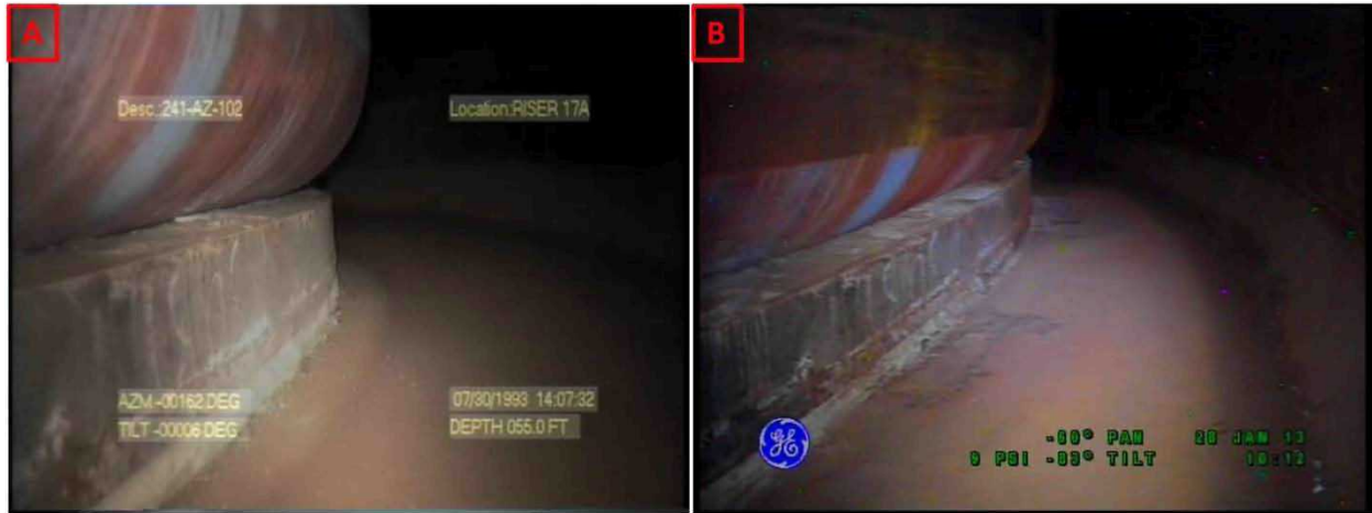
Figure 3-4. Riser 78 Lower Knuckle and Annulus Floor Comparisons Between Inspections on July 30, 1993 (A) and January 28, 2013 (B) Looking Towards Riser 90
