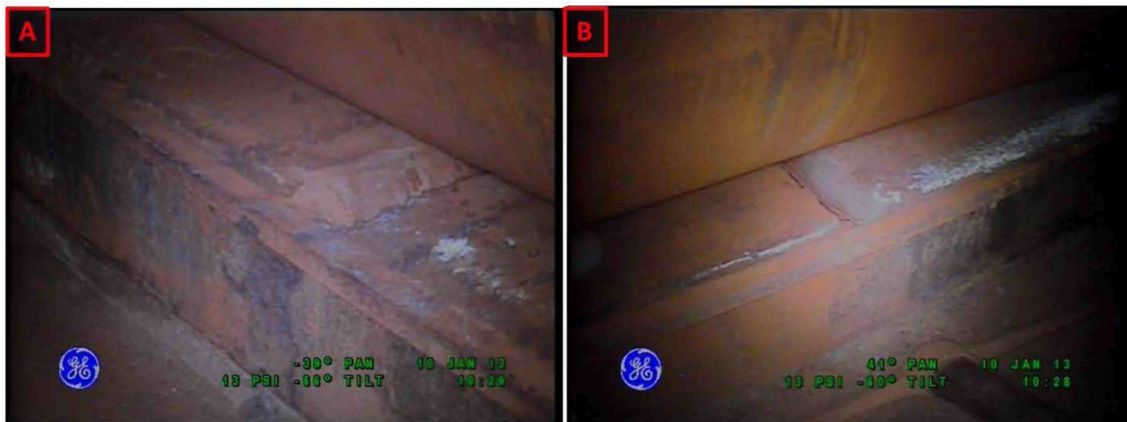
Figure 2-36. Riser 89 General Condition of the Refractory Slots on January 10, 2013
