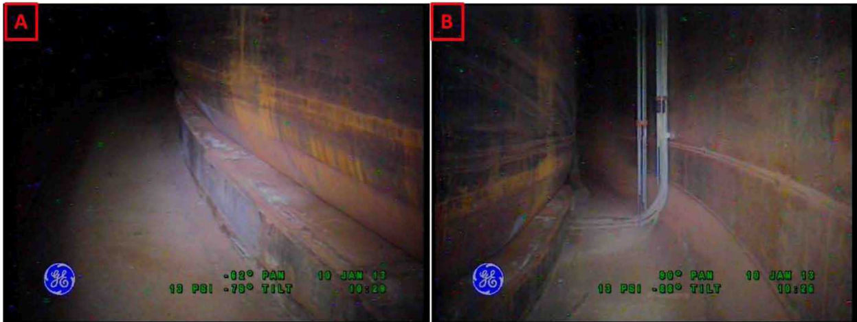
Figure 2-35. Riser 89 Lower Knuckle and Annulus Floor Condition on January 10, 2013 Looking Towards Riser 83 (A) and Looking Towards Riser 101 (B)
