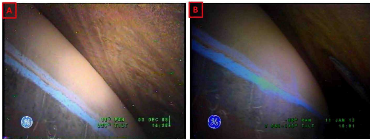
Figure 2-14. Riser 82 Upper Haunch Comparisons Between Inspections on December 3, 2008 (A) and January 11, 2013 (B) Looking Towards Riser 105
