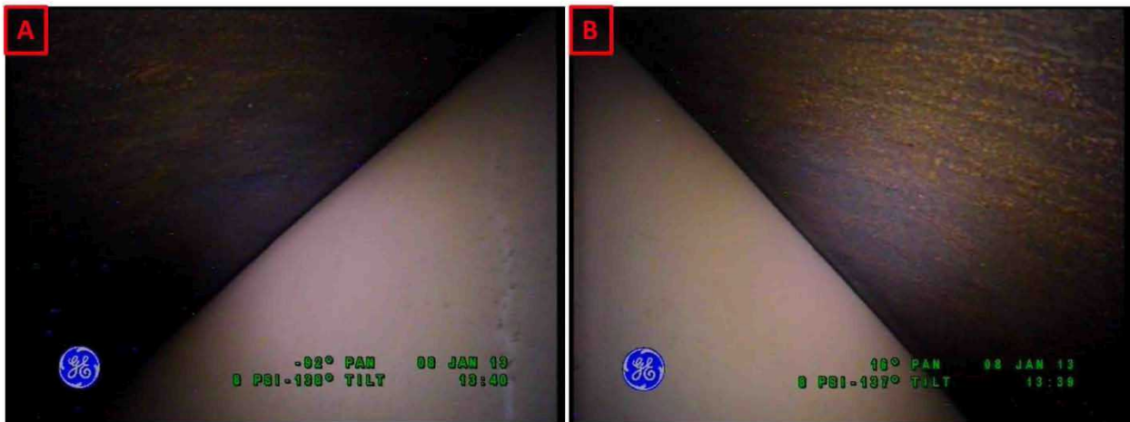
Figure 2-40. Riser 92 General Condition of the Upper Haunch on January 8, 2013 Looking Towards Riser 97 (A) and Looking Towards Riser 85 (B)
