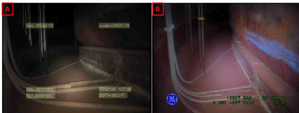
Figure 3-3. Riser 78 Lower Knuckle and Annulus Floor Comparisons Between Inspections on July 30, 1993 (A) and January 28, 2013 (B) Looking Towards Riser 93
