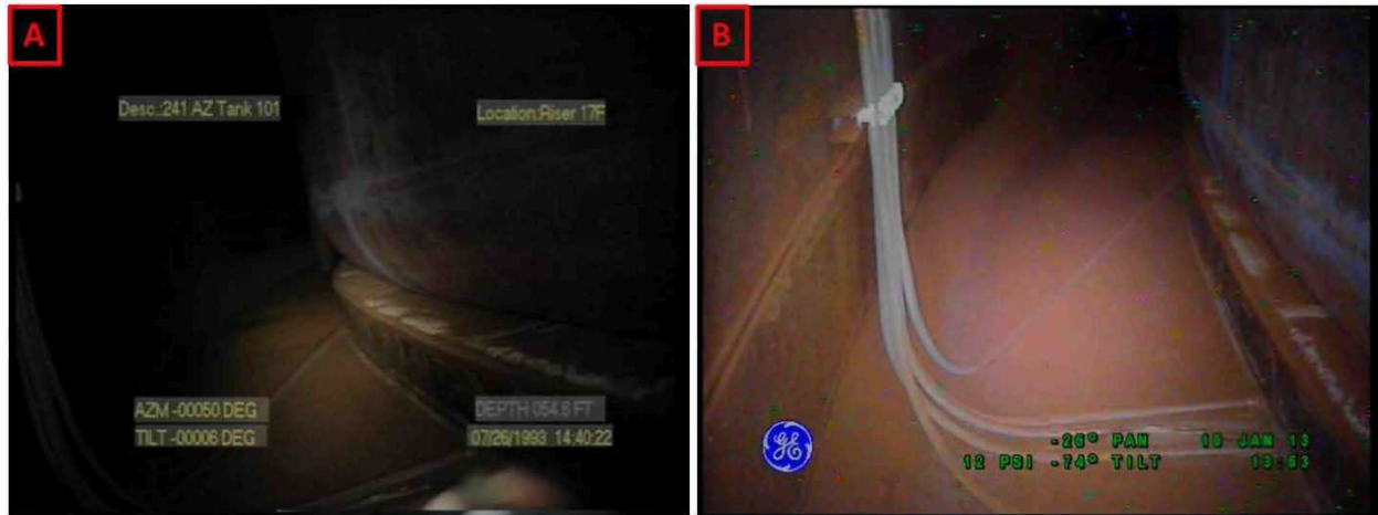
Figure 2-20. Riser 83 Lower Knuckle and Annulus Floor Comparisons Between Inspections on July 26, 1993 (A) and January 10, 2013 (B) Looking Towards Riser 96
