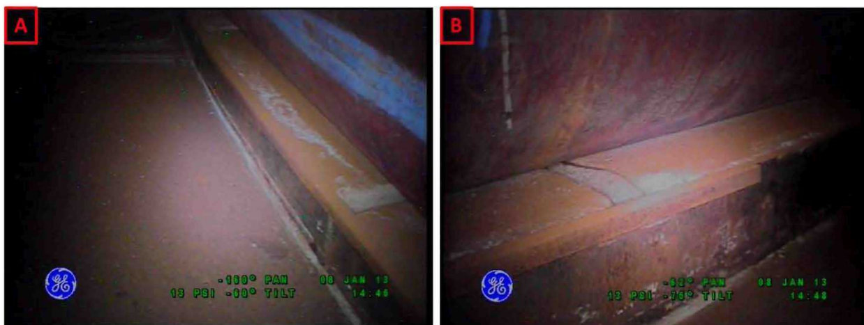
Figure 2-42. Riser 92 General Condition of the Refractory Slots on January 8, 2013
