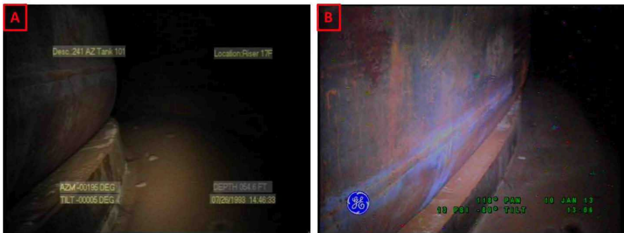
Figure 2-21. Riser 83 Lower Knuckle and Annulus Floor Comparisons Between Inspections on July 26, 1993 (A) and January 10, 2013 (B) Looking Towards Riser 89
