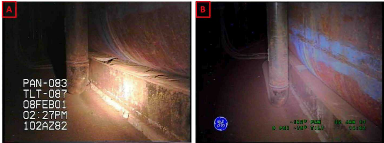
Figure 3-19. Riser 82 Lower Knuckle and Annulus Floor Comparisons Between Inspections on February 8, 2001 (A) and January 22, 2013 (B) Looking Towards Riser 95
