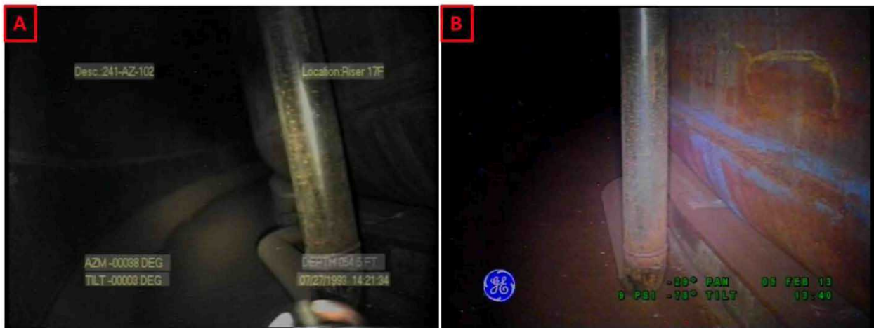
Figure 3-26. Riser 84 Lower Knuckle and Annulus Floor Comparisons Between Inspections on July 27, 1993 (A) and February 5, 2013 (B) Looking Towards Riser 85
