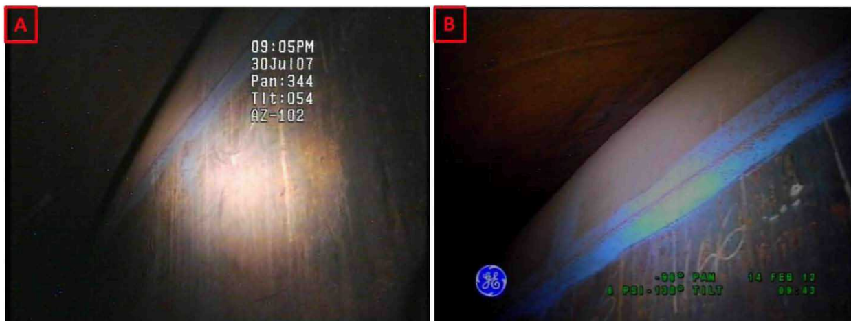
Figure 3-10. Riser 80 Upper Haunch Comparisons Between Inspections on July 30, 2007 (A) and February 14, 2013 (B) Looking Towards Riser 91
