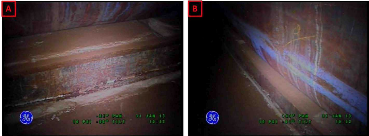
Figure 3-31. Riser 86 General Condition of the Refractory Slots on January 31, 2013
