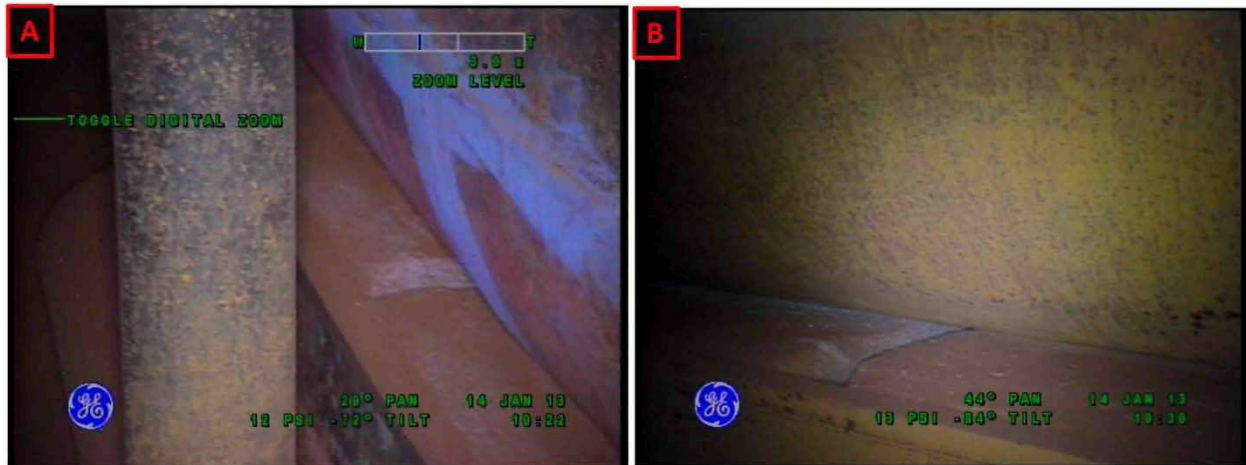
Figure 2-25. Riser 84 General Condition of the Refractory Slots on January 14, 2013
