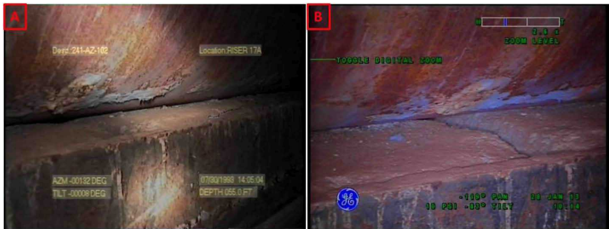
Figure 3-5. Riser 78 General Condition of the Refractory Slots on July 30, 1993 (A) and January 28, 2013 (B)
