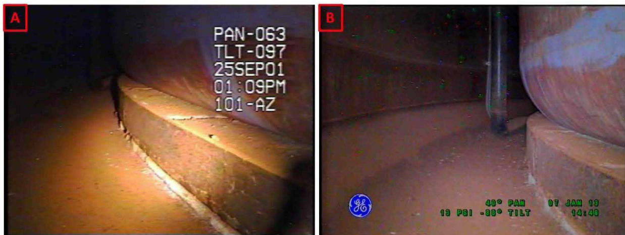
Figure 2-28. Riser 86 Lower Knuckle and Annulus Floor Comparisons Between Inspections on September 25, 2001 (A) and January 7, 2013 (B) Looking Towards Riser 87
