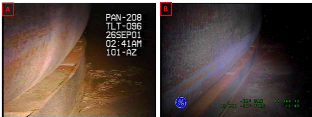
Figure 2-16. Riser 82 Lower Knuckle and Annulus Floor Comparisons Between Inspections on September 26, 2001 (A) and January 11, 2013 (B) Looking Towards Riser 105
