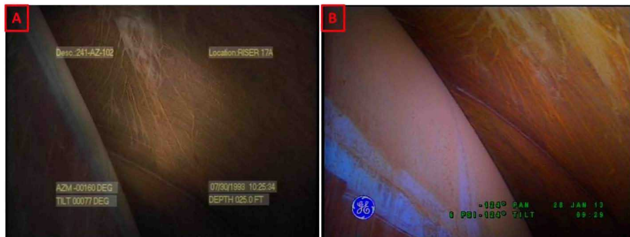
Figure 3-2. Riser 78 Upper Haunch Comparisons Between Inspections on July 30, 1993 (A) and January 28, 2013 (B) Looking Towards Riser 90
