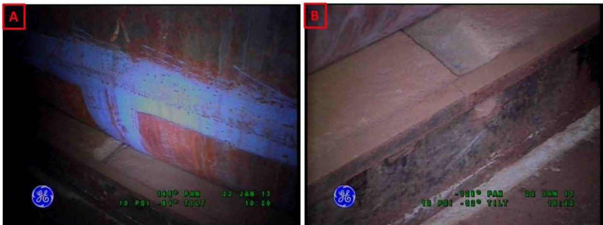
Figure 3-17. Riser 81 Lower Knuckle and Annulus Floor Condition on January 22, 2013
