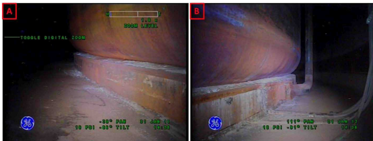
Figure 3-33. Riser 88 Lower Knuckle and Annulus Floor Condition on January 31, 2013 Looking Towards Riser 90 (A) and Looking Towards Riser 104 (B)
