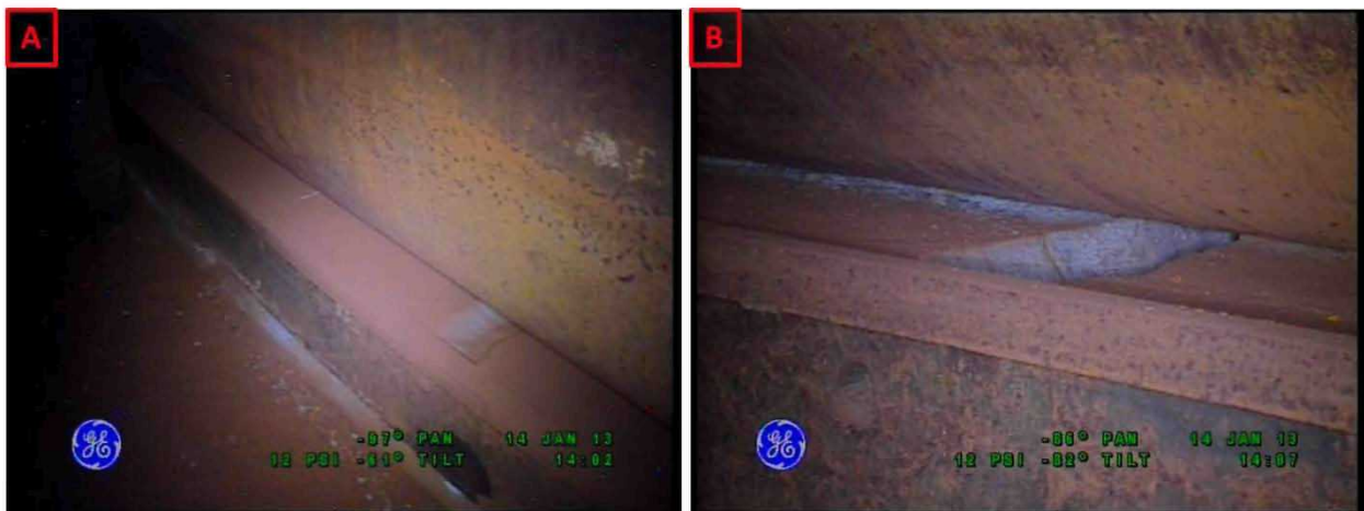
Figure 2-9. Riser 79 General Condition of the Refractory Slots on January 14, 2013
