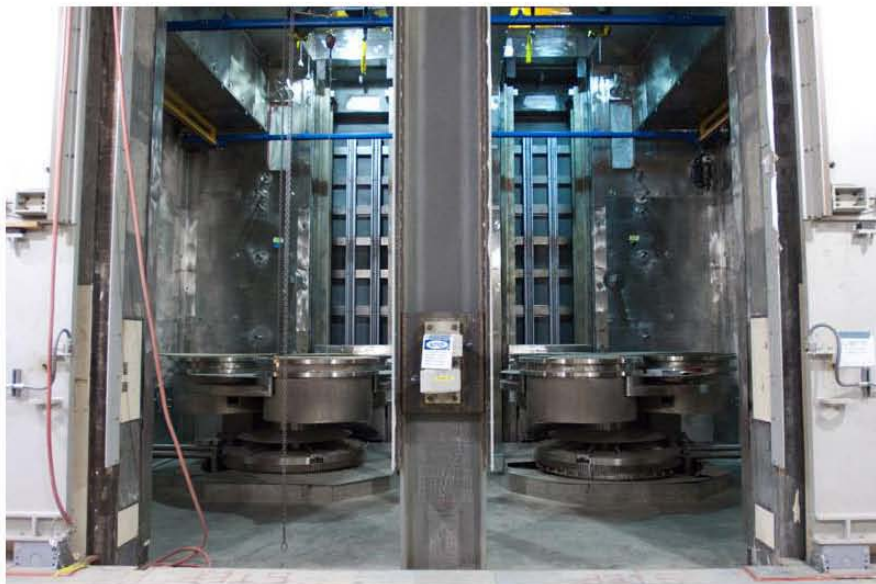
Figure 2-8. Canister Turntables beneath LAW Melter Discharge Chambers
