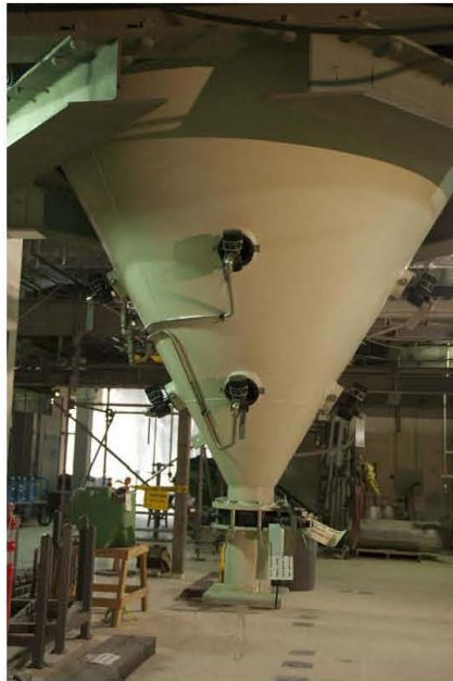
Figure 2-5. Glass Former Feed Hopper (WTP LAW facility March 2010)
