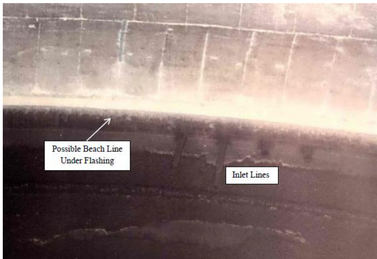
Figure 4-7. Tank C-101 Photograph February 13, 1970 (700695-4 CN)
