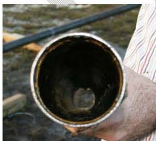
Figure 27. Unplugged 8 ft Bentonite plug at 310 ft pipeline (top). Unplugged blockage section (bottom).
