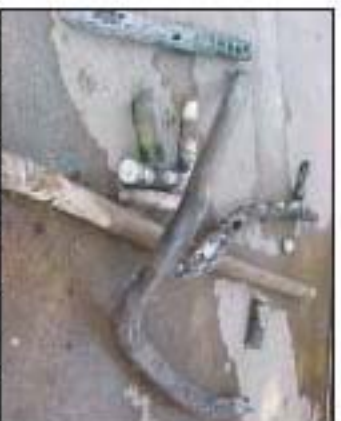
Top photo, foulant exits a pipe during Hydrokinetics cleaning. Bottom photo, foulant comes out in a snake-like fashion.
