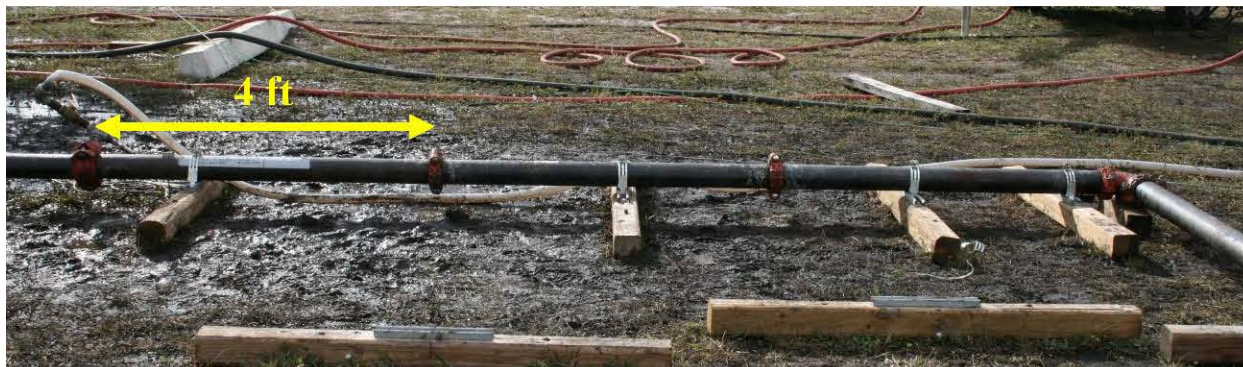
Figure 10. 12 ft long Bentonite based blockage section.
