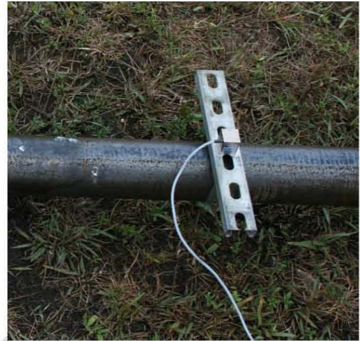
Figure 7. Installation of accelerometer on the pipeline.
