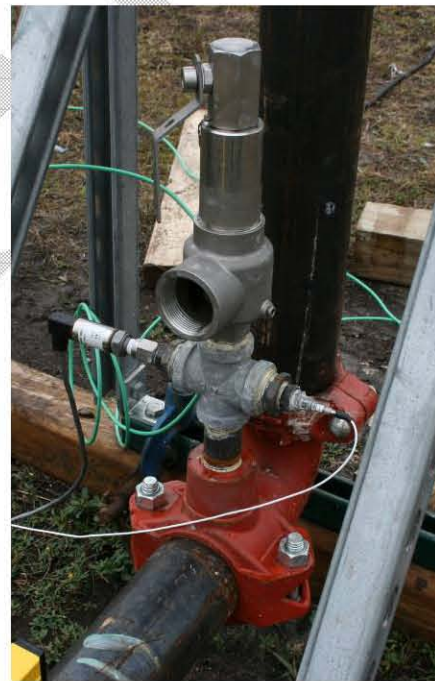
Figure 5. Pressure relief valve at inlet (300 psi).
