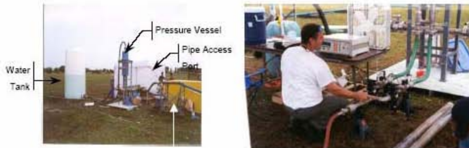
Fig. 15. Equipment and control module used in the FIU demonstration of the AEA Technology Fluidic Wave Action process. Source: M.A. Ebadian, Plugging Prevention and Unplugging of Waste Transfer Pipelines, Part 1-Equipment Tests of Blockage Locating, Detecting, and Unplugging Technologies on the Full-Size Test Beds , HCET-1998-M004-001-04, Hemispherical Center for Environmental Technology, Florida International University, 2002.
