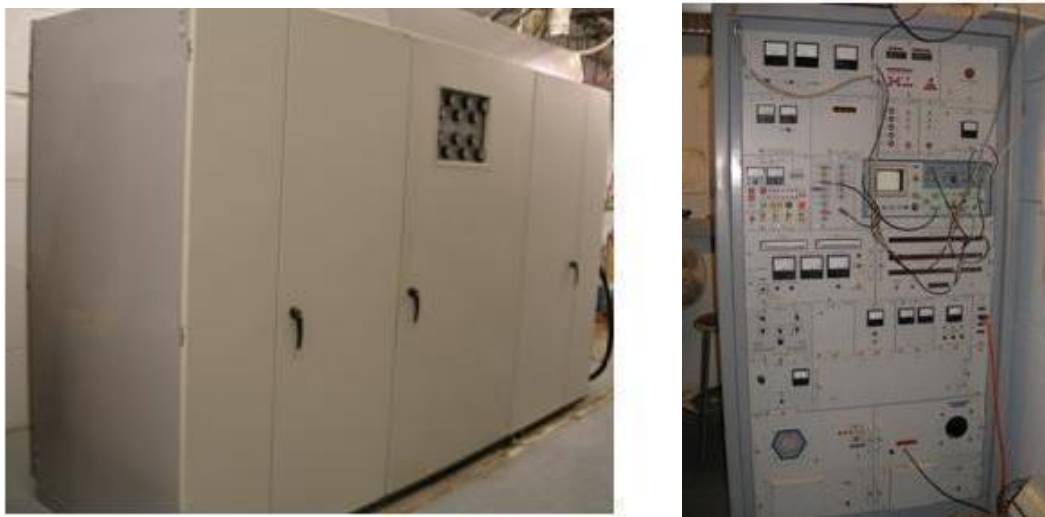
Figure 22. Available 65-MW modulator (left), and its control rack (right).
