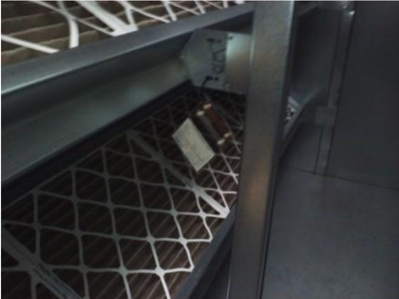
Figure 7 - Typical Coupon Mounting - Example Shown is Immediately Downstream of Supply Air Filters as Found in Large Roof Top Fan Units
