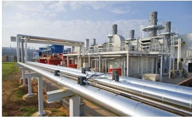
BMW Methane Facility at Spartanburg Facility
