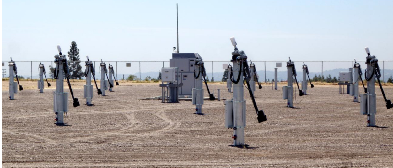
Figure 8-3. CSUN site prepared for panel mounting. Note the helical piles are topped with trackers and attached junction boxes
