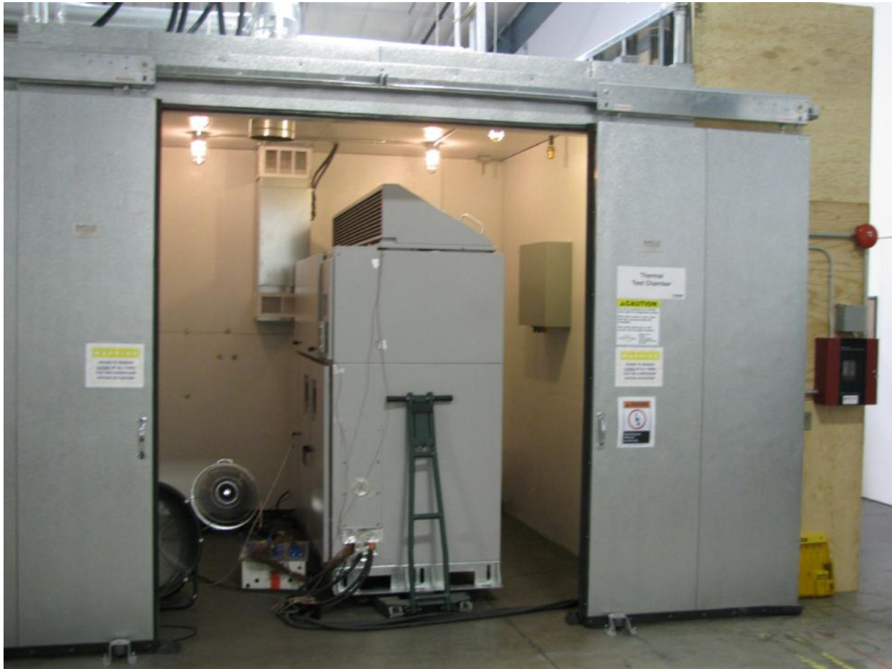
Figure 7-27. A 260kW inverter prototype wired up within a thermal test chamber within PV Powered's new engineering facility.
