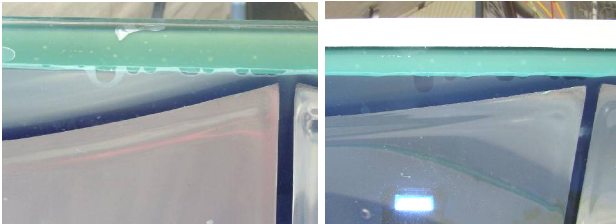
Fig. 26-a,b: Adhesive de-bond with water inside and field repair after pressure spray wash.
