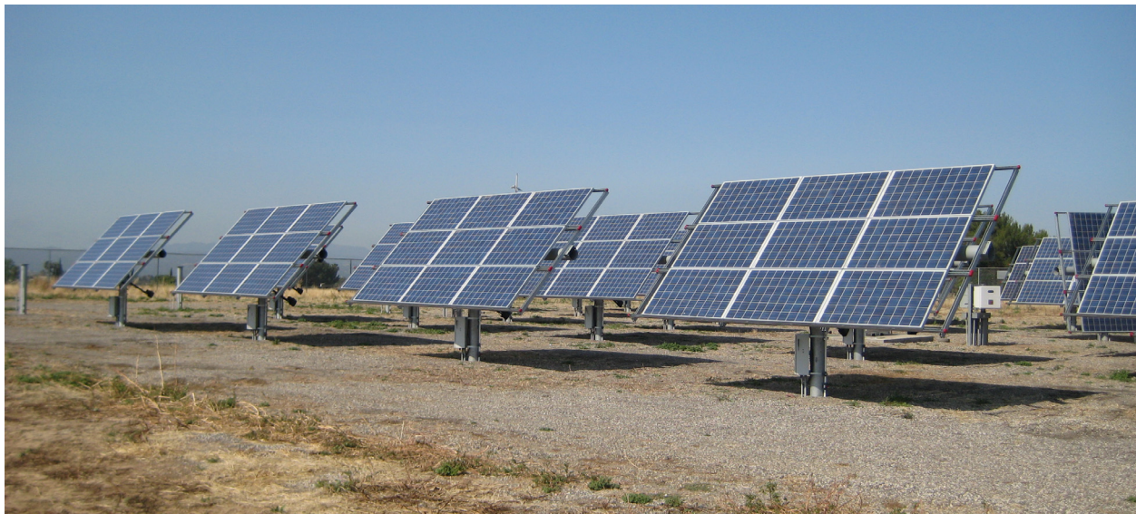
Figure 8-20. CSUN Power Plant After Retrofit With Flat PV Panels.
