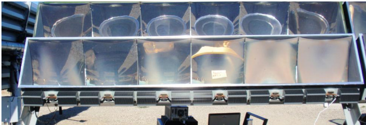
Figure 8-13. Preferential mirror discoloration near the right hand side adjacent to the module vent.
