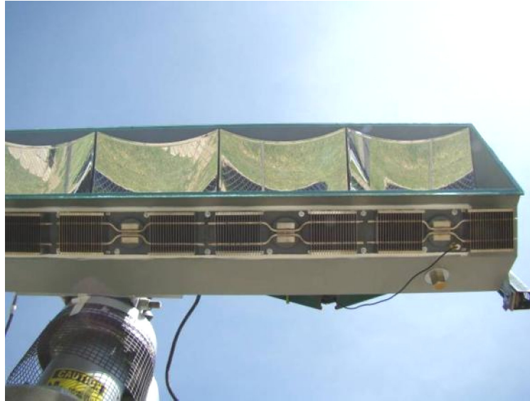
Fig. 15-b: Heat sinks and receiver wall
