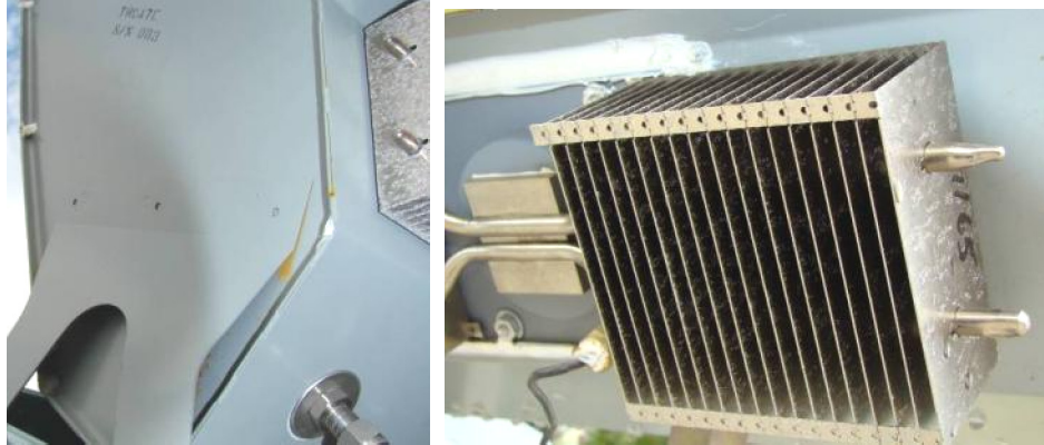
Fig. 27-a,b: Observed minor corrosion on heat sinks and POC chassis.
