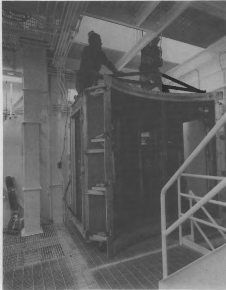
Figure 3. Rigid Portable Greenhouse that Connects to the Generator During Sectioning Operations
