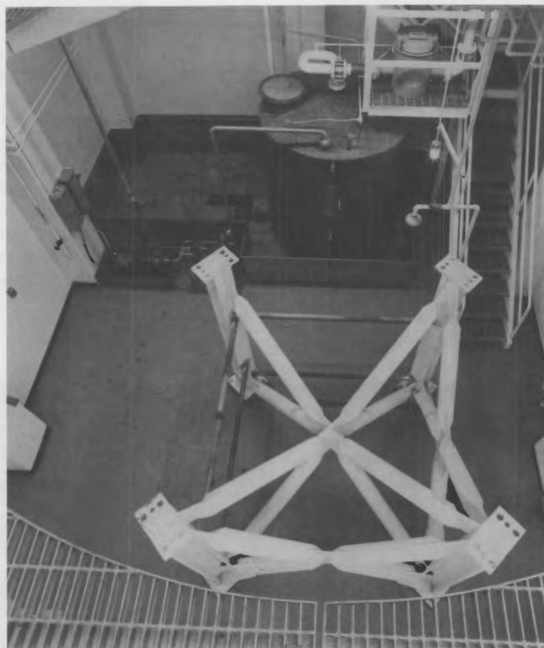
Figure 2. View of the Stand for Supporting the Steam Generator in the SGEF Tower. The liquid radioactive waste handling system is shown in the background.
