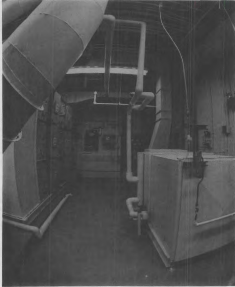
Figure 4. SGEF Equipment Room
