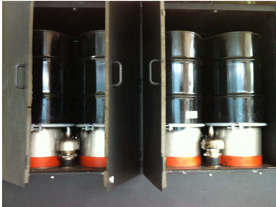
Figure 9-12: Filter box with doors open. Bags are inverted inside barrels by syngas flow
