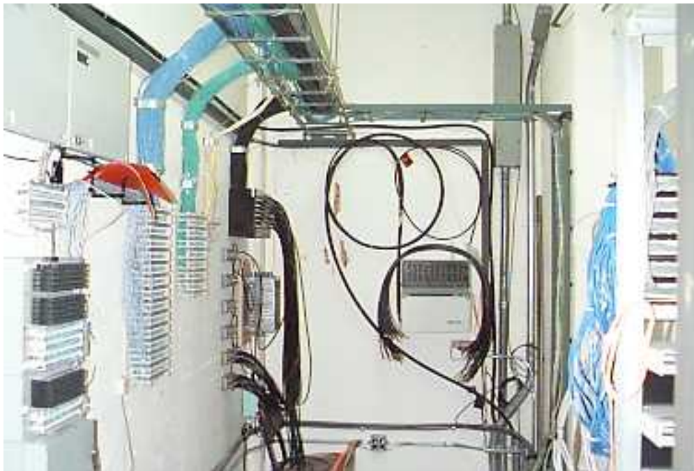
Figure 9.11. A Wiring Closet in a Commercial Building that Includes the Telephone Exchange Wiring (left hand side), Coaxial-Cable Based Broadband Satellite TV Distribution Wiring (further along left hand side), a Fiber Optic Video Distribution Network (far wall), and a 96 Port Ethernet Distribution Network (right hand side). Each communication network has independent wiring and shares the cable trays and building risers.
